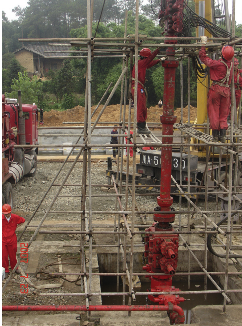
Figure 8.4 Blowout preventer at the wellhead.
