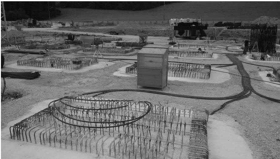
Figure 16.8 Pipe network between the groups of energy geostructures and the manifolds. Image courtesy: Marti Construction.
