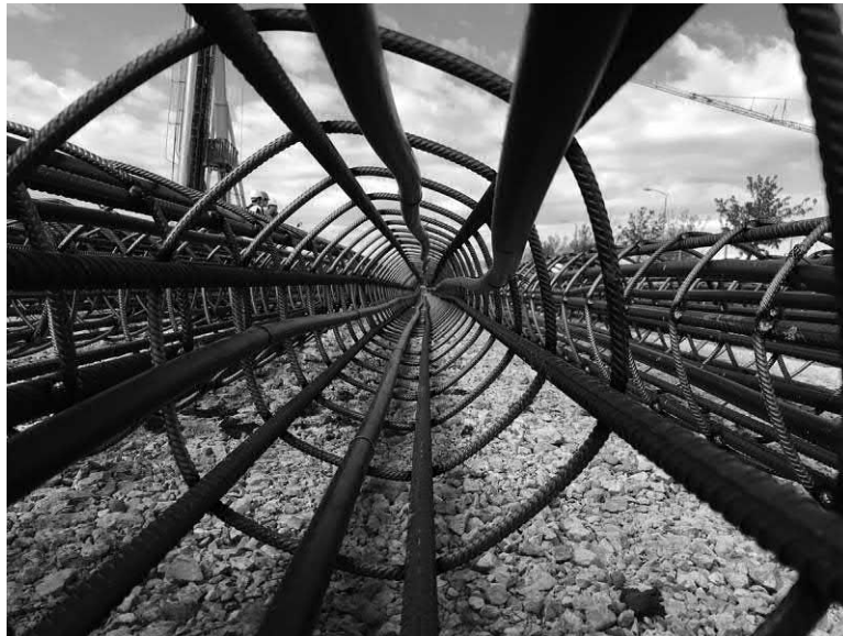
Figure 16.3 Pipe fixing on the inside of the reinforcing cage of an energy pile.
