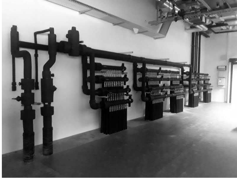
Figure 16.9 Technical room where all manifolds arrive when the system is ready for connection to the heat pump. Image courtesy: Marti Construction.
