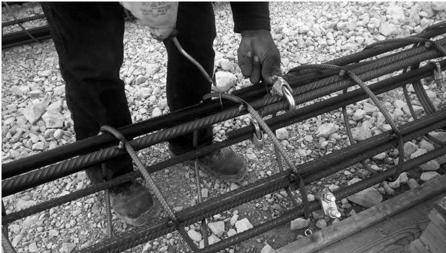
Figure 16.4 Use of wire ties to fix the pipes to an energy pile.
