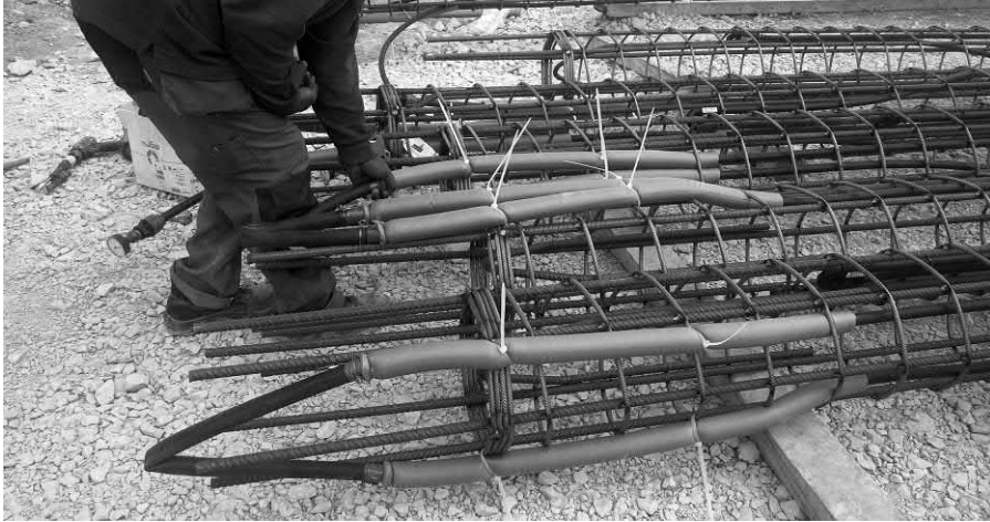
Figure 16.5 Protection of the inlet and outlet of pipes at the head of energy piles by a plastic connection (characterised by a black colour in the figure) to avoid any damage during concreting.
