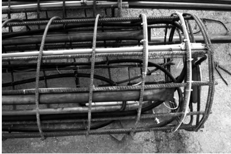
Figure 16.1 Example of pipe bending at the edge of an energy pile.
