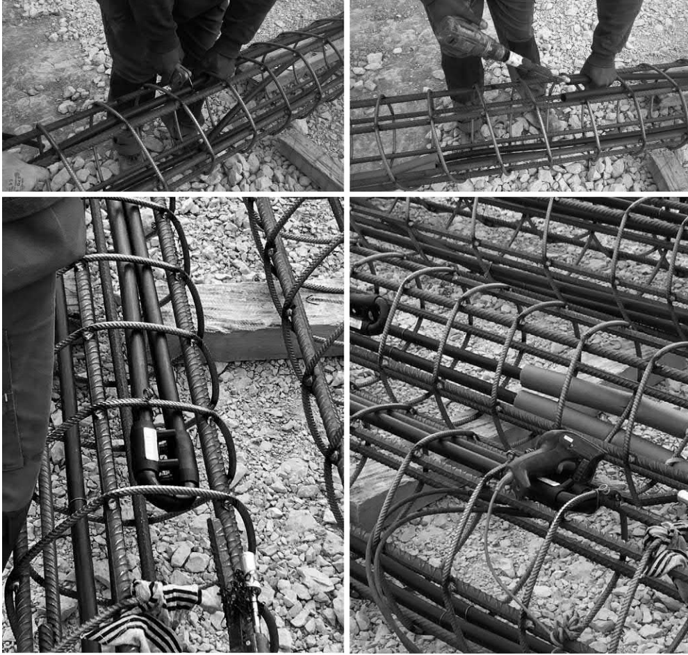
Figure 16.2 Example of the connection of pipes at their edge through thermally welded U-bends in an energy pile.
