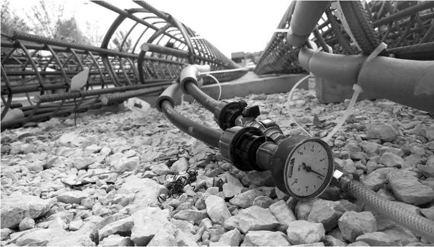
Figure 16.10 Manometer placed at the end of pipe loops to control the pressure at any time during the construction.
