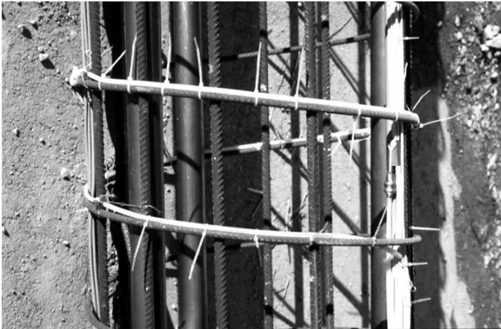
Figure 14.30 Attachment of optical fibres to the reinforcing cage of an energy pile to measure its radial strains.
