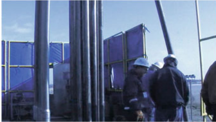
(k) Lifting the inner tube from the ground through the catwalk to the rig floor
