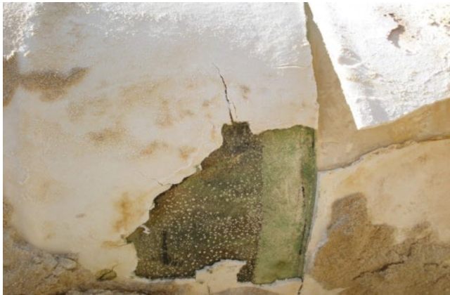
Figure 9.4 Failure of a flame-sprayed PP field joint coating on a three-layer PP-coated gas pipeline.
