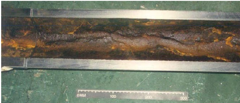
Figure 11.3 Groove corrosion promoted by microbial activity. Source: [2].
