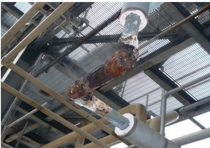
Figure 13.7 Isolated CUI of piping with expanded pearlite insulation.
