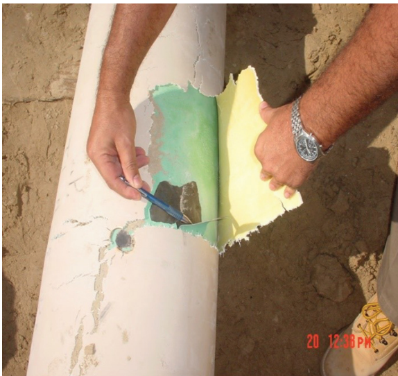
Figure 9.3 Cracking and disbondment of the three-layer PP coating due to thermo-oxidative degradation.
