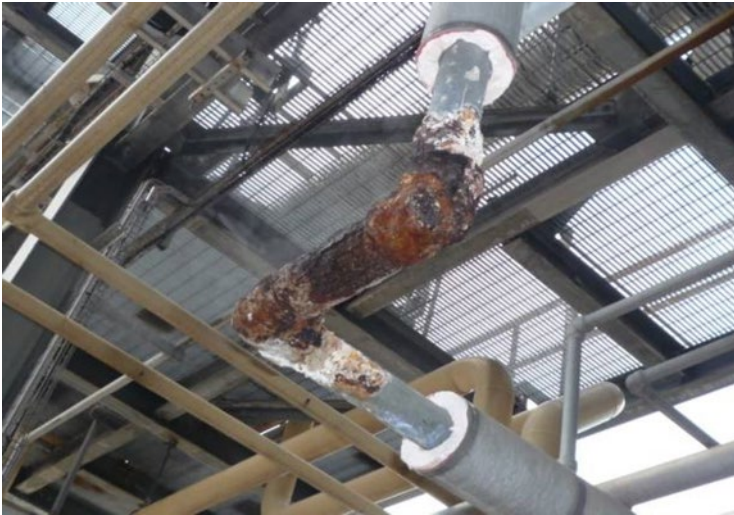
Figure 13.7 Isolated CUI of piping with expanded perlite insulation. (see colour plate section).
