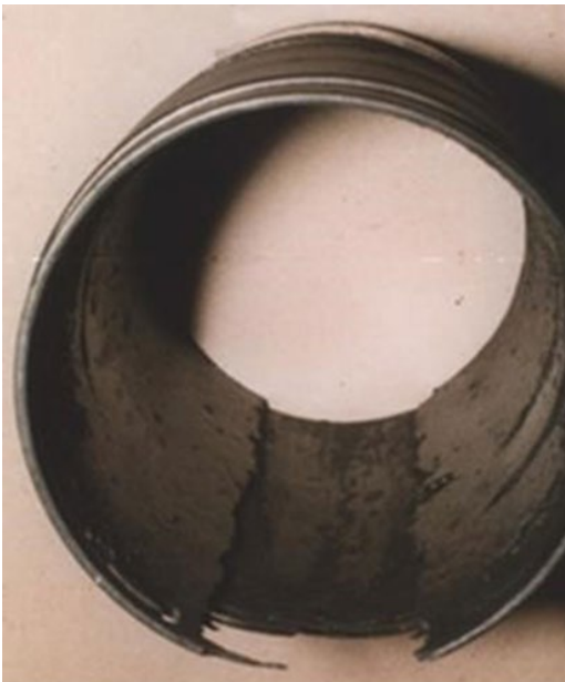
Figure 17.2 An example of bottom of line groove corrosion. (see colour plate section).
