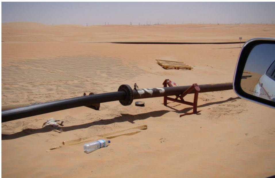
Figure 9.7 Field insertion of HDPE liner in a steel flowline. (see colour plate section).
