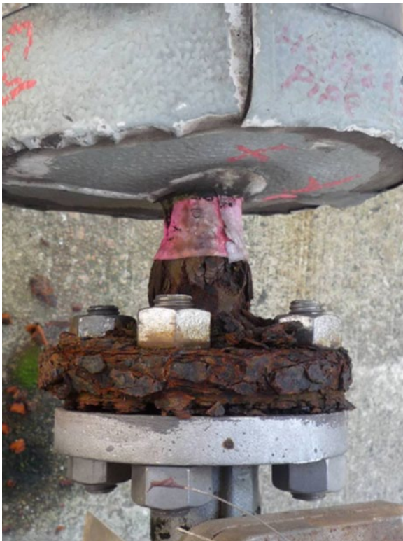
Figure 13.6 A typical example of carbon steel sweating CUI damage accelerated by galvanic corrosion at a carbon steel/stainless steel flange material specification change. (see colour plate section).
