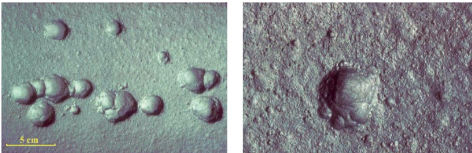
Figure 11.2 Localised hemispherical damage. (see colour plate section).
