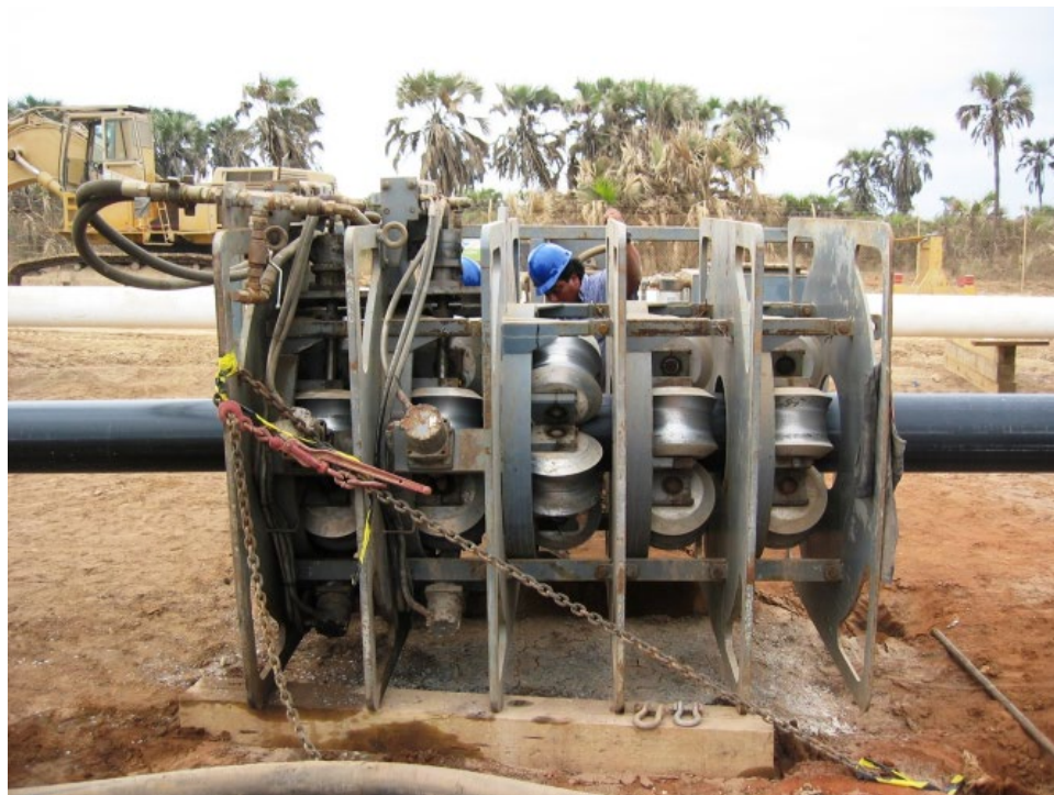
Figure 15.4 An example of roller box reduction equipment. (see colour plate section).
