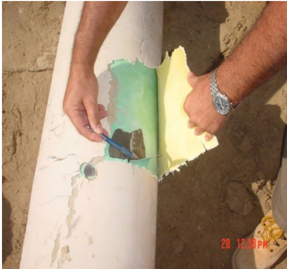
Figure 9.3 Cracking and disbondment of the three-layer PP coating due to thermo-oxidative degradation. (see colour plate section).
