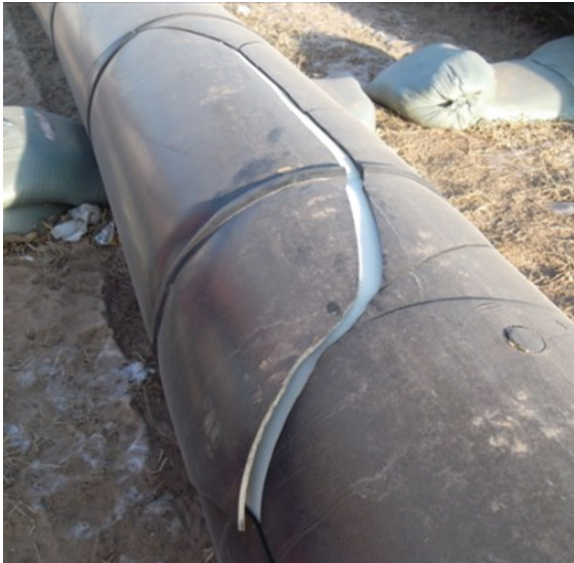
Figure 9.2 Completely disbonded three-layer PP coatings removed from a gas pipeline.
