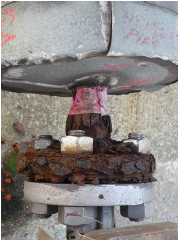
Figure 13.6 A typical example of carbon steel sweating CUI damage accelerated by galvanic corrosion at a carbon steel/stainless steel flange material specification change.
