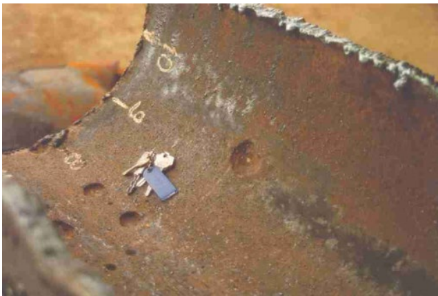
Figure 11.1 Typical features of MIC type damage characteristic of localised morphologies.
