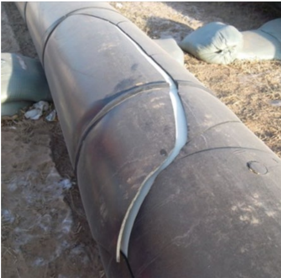
Figure 9.2 Completely disbonded three-layer PP coatings removed from a gas pipeline (see colour plate section).
