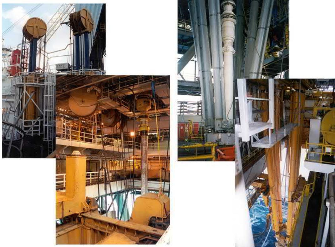
FIG. 5.28 Wire and hydraulic in line deepwater tensioning systems. Source: Kingdom Drilling training 2009.
