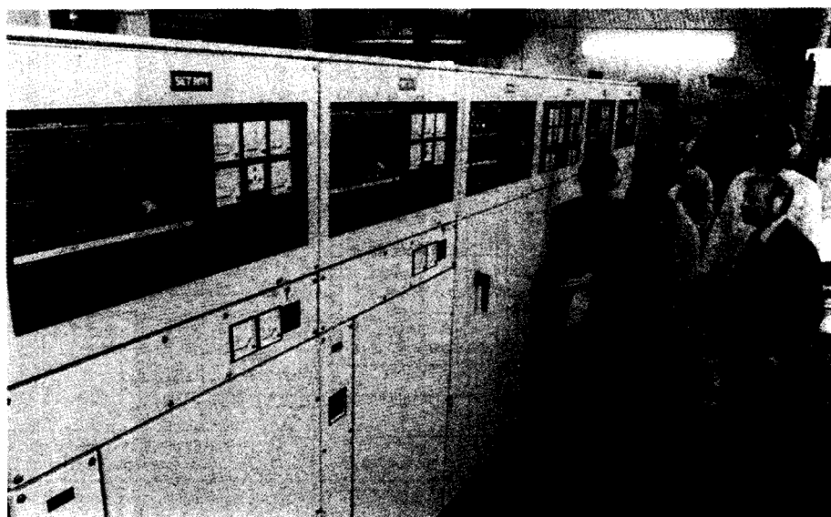
Figure 9.59 A four generator set cubicle suite, incorporating switchgear and control gear, on test at the manufacturer's works (Courtesy: Petbow Ltd)
