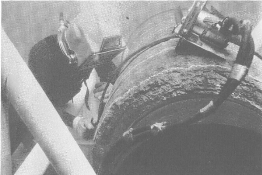
FIG. 18–3 This diver/welder is performing a wet-stick weld repair on a platform in the Gulf of Mexico. (Courtesy Chicago Bridge and Iron/SeaCon Services)
