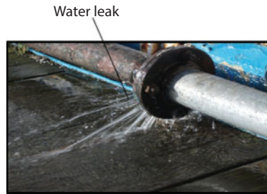
Figure 2.5 Water leaking from a water supply well casing.
