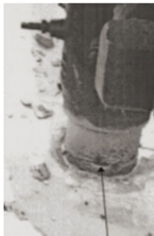
Figure 2.3 Damaged surface casing on an water injection well (Farooqui, 1998).
