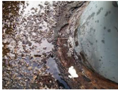
Figure 2.4 Pitted surface casing of a oil well (Farooqui, 1998).
