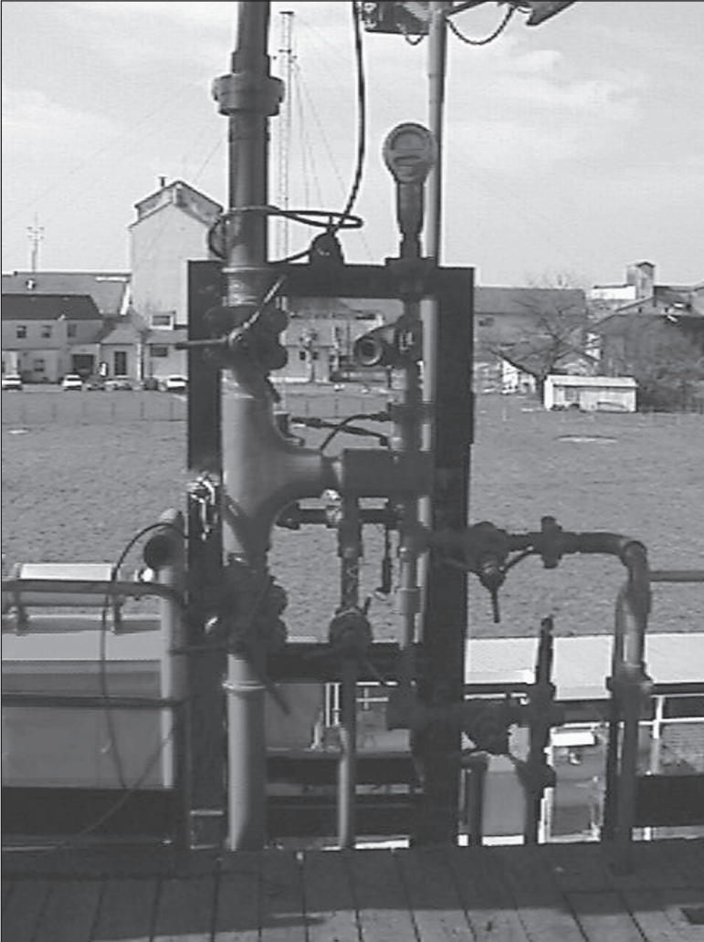
Fig. 5–13. Standpipe manifold on a land rig
