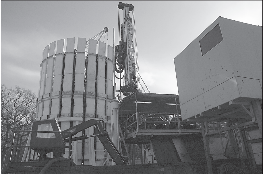
Fig. 5–3. The Larchford Drillmaster automated singles rig, drilling in the south of England
