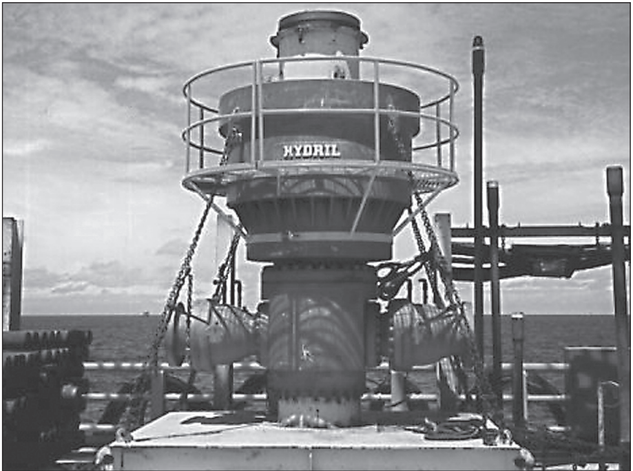
Fig. 11–12. Diverter with large-diameter side outlets
