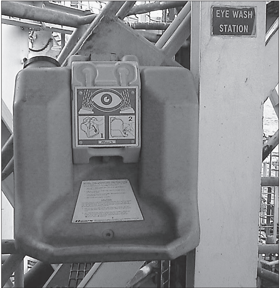
Fig. 14–3. Eyewash station, positioned around the rig
