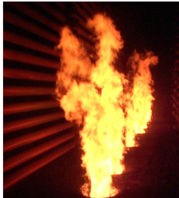
Figure 8.8 Poor flame pattern from the first burner.
