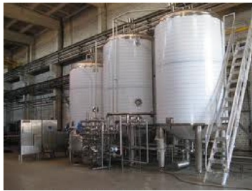
Vertical storage tanks with legs
