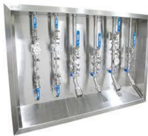
Hose Station in Chemical Plant
