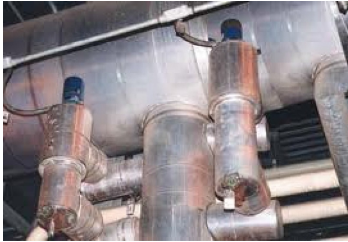
Photo of Drip Leg on Steam Line
