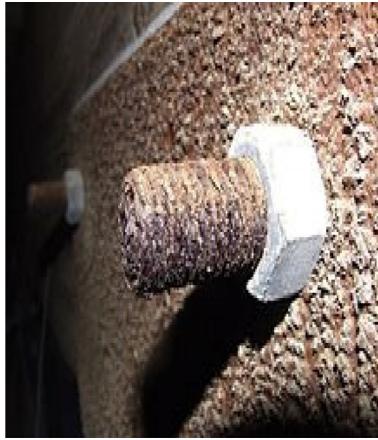
Corrosion on exposed metal
