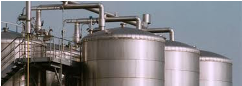
Access platform at vertical storage tanks
