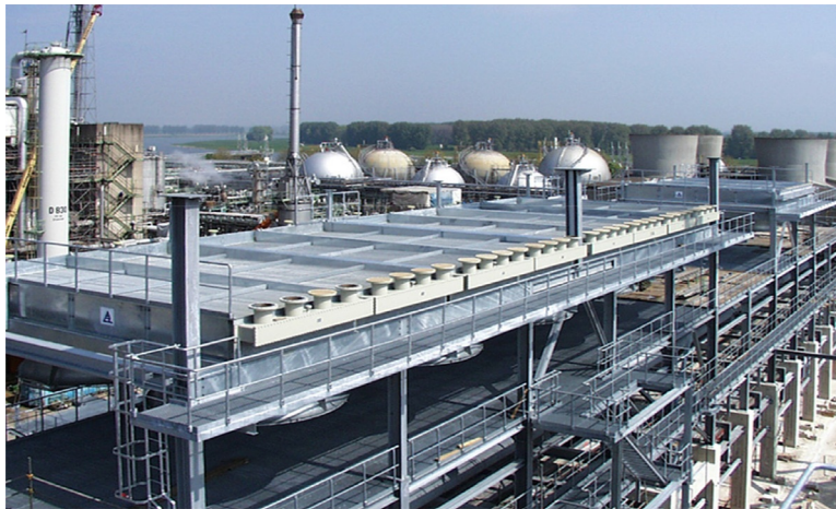
Photo of air cooler on a pipe rack in a process plant
