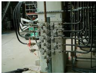
Steam Tracing Manifold at Column
