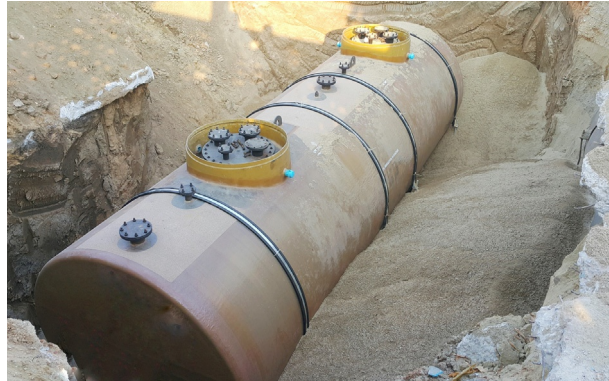
Typical buried petroleum tank at gas station
