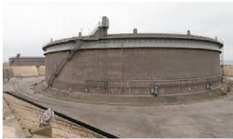
Tank farm storage on berm
