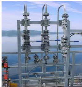
Hose Station at Platform
