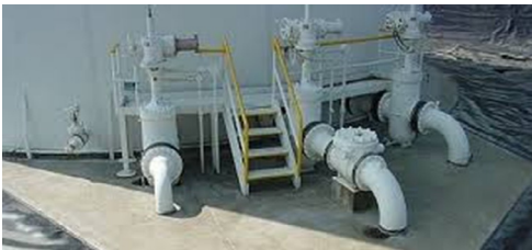
Bottom outlet platform
