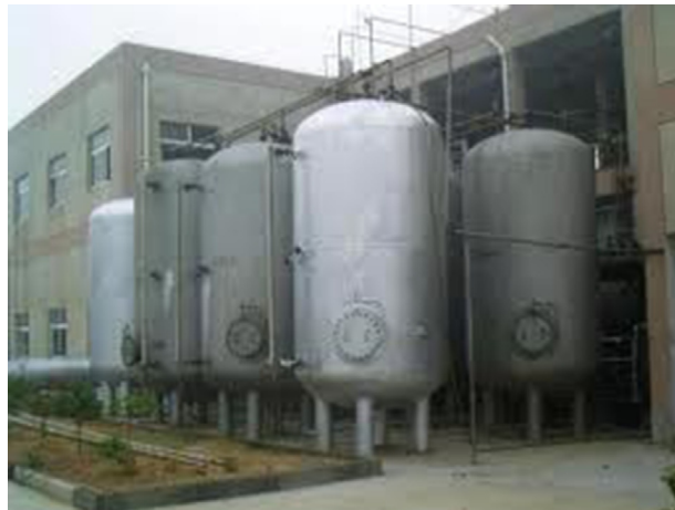
Photo of intermediate storage tanks
