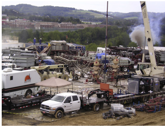
FIGURE 2.8 Hydraulic fracturing operation underway on two Marcellus Shale wellheads in southwestern Pennsylvania. Pump trucks are on the right, blender and manifold in center, proppant sand in left background with two men on tank, monitoring and control trailer to left. Water supply was in a large impoundment behind photographer. Photograph by Dan Soeder.
