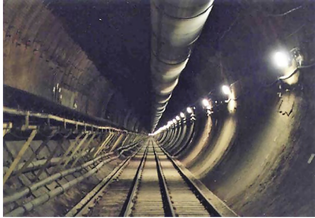
FIGURE 7.1 The North Ramp of the Exploratory Studies Facility (ESF) tunnel under Yucca Mountain, Nevada. This U-shaped tunnel into and out of the mountain is five miles (8 km) in length and 25ft (7.6 m) in diameter.
