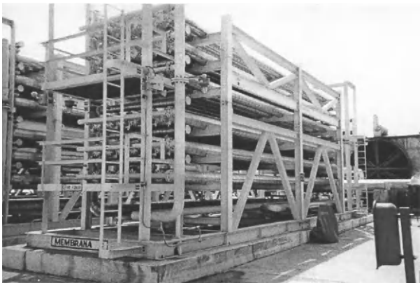
FIGURE 1-16 Horizontal membrane skid.
