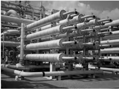
FIGURE A-8 Skid containing Air Liquide membrane elements.
