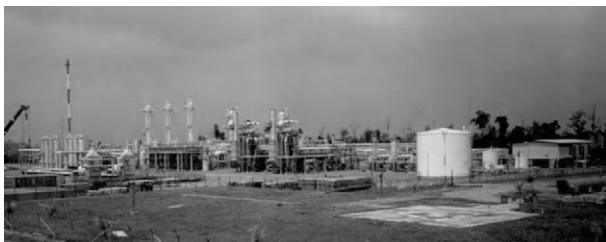
FIGURE A-1 Grissik gas plant.
