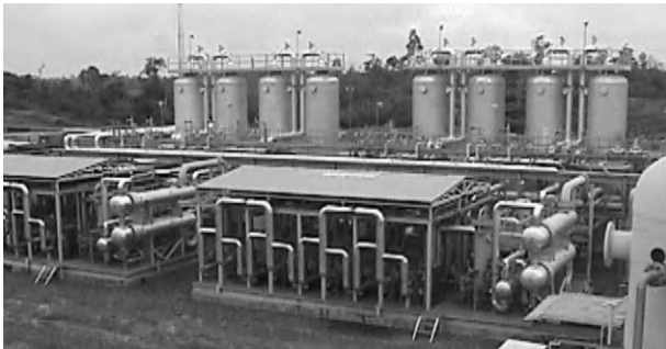
FIGURE A-3 Engelhard thermal swing adsorption unit.
