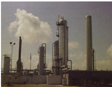
FIGURE B-3 Amine Sweetener includes a contactor, regenerator and a BTEX stripper.
