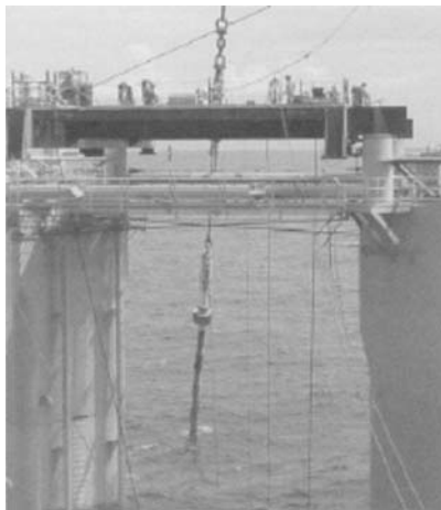
Figure 9.64 The Prince SCR during hang-off installation showing the pre-installed VIV strakes [Gore and Mekha, 2002]
