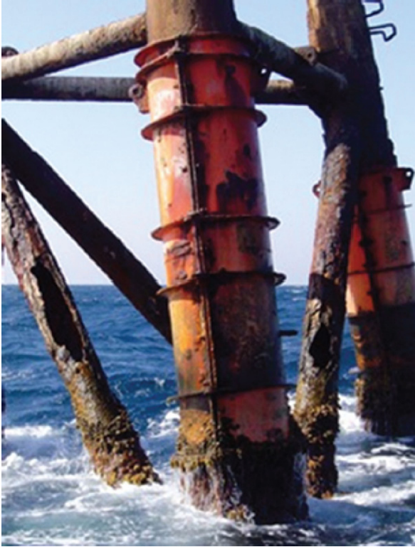
Figure 8.4 Corroded bracing. Source: Figure reproduced from El-Reedy, 2012, Fig. 7.47 .
