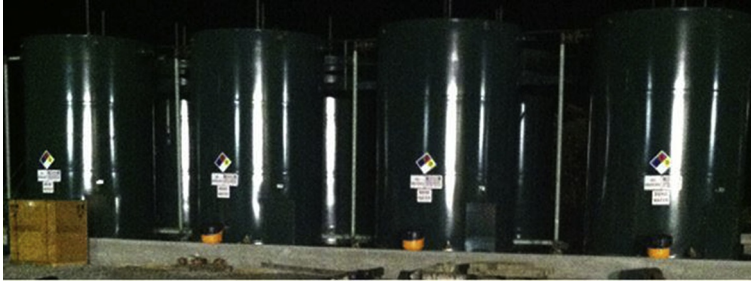
Fig. 12.12 Oil tanks (upright tanks).
