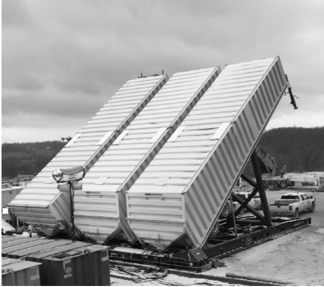
Fig. 16.5 Sand storm system.
