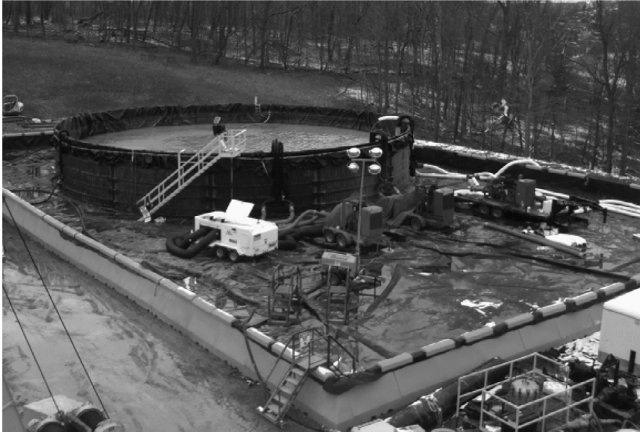
Fig. 16.2 Aboveground storage tank (AST).
