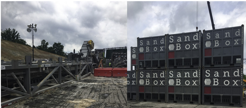
Fig. 16.6 Sand box system.
