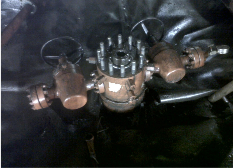
Figure 16.22 Tubing head with production tubing hung inside the tubing hanger.
