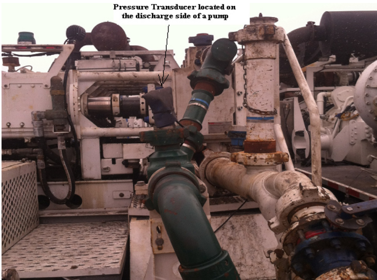
Figure 16.21 Pressure transducer on a pump.
