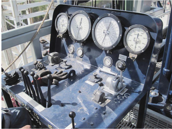
■ FIG. 3.32 Rig-assist control panel. (Courtesy of International Snubbing Services.)
