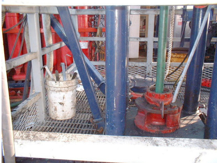
■ FIG. 5.21 ESP power cable installation in work window. (Courtesy of International Snubbing Services.)
