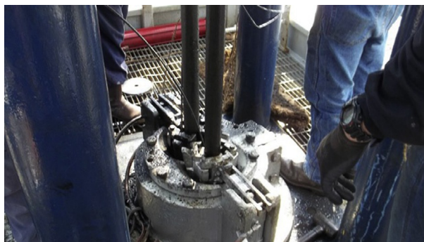
■ FIG. 5.6 Dual stationary slips in window. (Courtesy of International Snubbing Services.)
