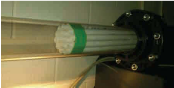
Figure 14.6. Upstream flow straighteners create uniform conditions.
