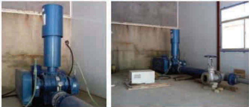
Figure 1.5k. Water-cooled air blower with separate power source.
