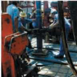
Assembly of the RAB tool at the FZDMS facility.
