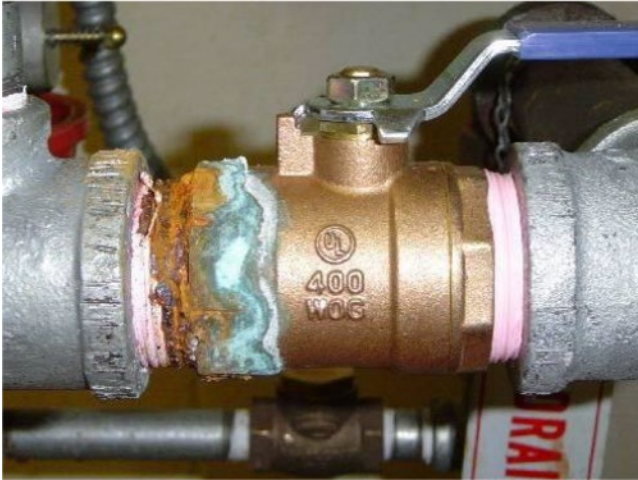
Figure 5.6 Galvanic corrosion of galvanized piping in connection with bronze valve.
