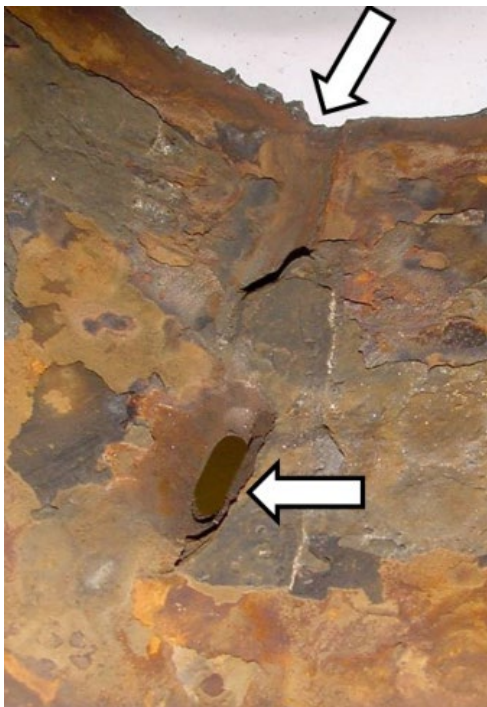
Figure 5.104 Channeling or six o'clock corrosion at the bottom of a gathering line. Arrows point to leak (bottom arrow) and profile. Note that the rust scale hides the channel for most of the distance between the two arrows.
