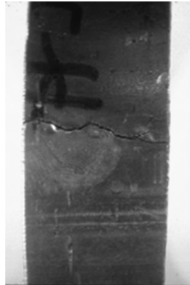
Figure 5.82 Stress corrosion cracking underneath insulation on a stainless steel condensate line. Source: Courtesy of NACE International.
