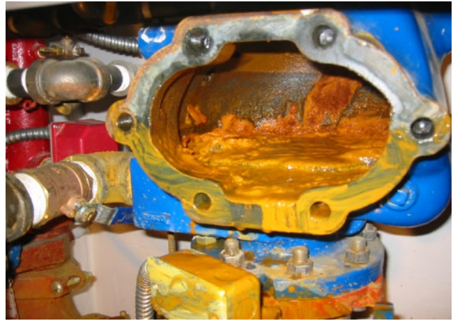
Figure 8.40 Corrosion at a control valve in a “dry” fire sprinkler system. Source: Photo courtesy Mark Hopkins, Hughes Associates, Baltimore, MD.
