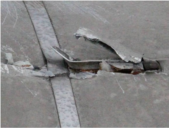
Figure 3.18 Mechanical damage to insulation jacketing.
