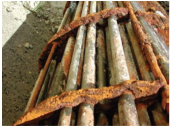
Figure 5.8 Titanium tubes in a cooling water heat exchanger with carbon steel baffles and water box. Deposits on the titanium tubes are the salts (scale) formed from the cooling water, and not corrosion [19]. Source: Reproduced with permission of Springer.
