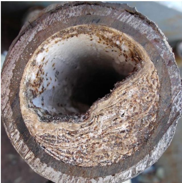
Figure 3.39 Boiler scale in steam generating piping.
