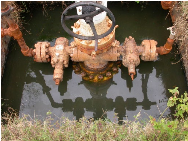
Figure 6.31 Wet valves in a sump on a crude oil pipeline.
