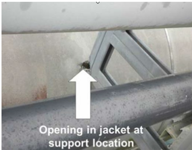
Figure 7.5 Torn thermal insulation jacketing due to motion of the structural supports on the piping.
