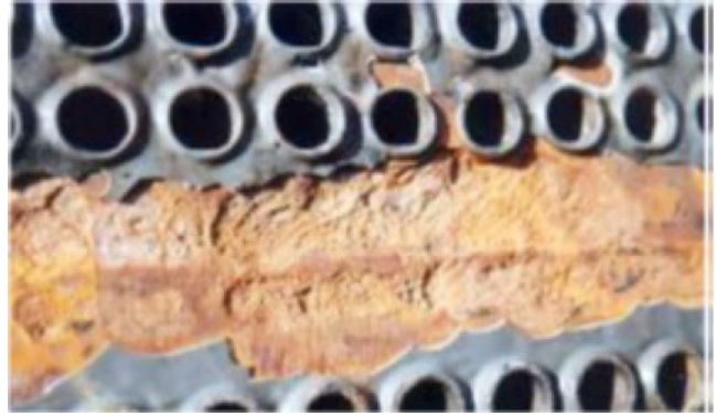
Figure 5.7 Painted carbon steel tube sheet in a heat exchanger with copper-alloy tubes [19]. Source: Reproduced with permission of Springer.
