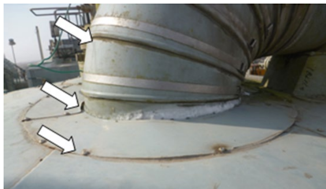
Figure 8.69 Locations where seams in insulation jacketing can lead to moisture ingress and corrosion.
