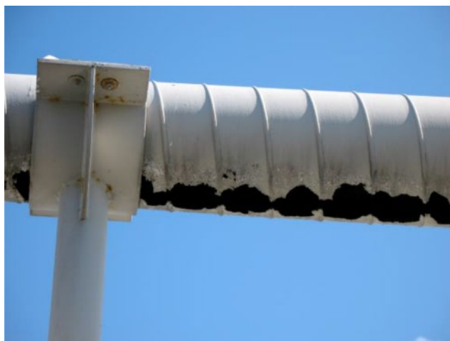
Figure 4.56 Aluminum corrosion at the six o'clock position where acidic atmospheric condensate water collected in a low-temperature ventilation system.
