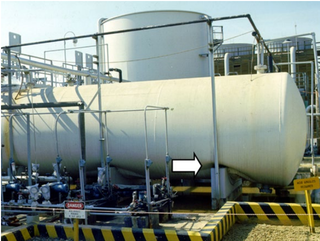
Figure 7.22 Slumping storage tank due to wall thinning.
