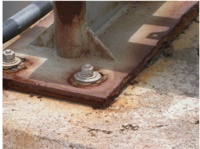
Figure 5.10 Corrosion of carbon steel structure connected to stainless steel fasteners.
