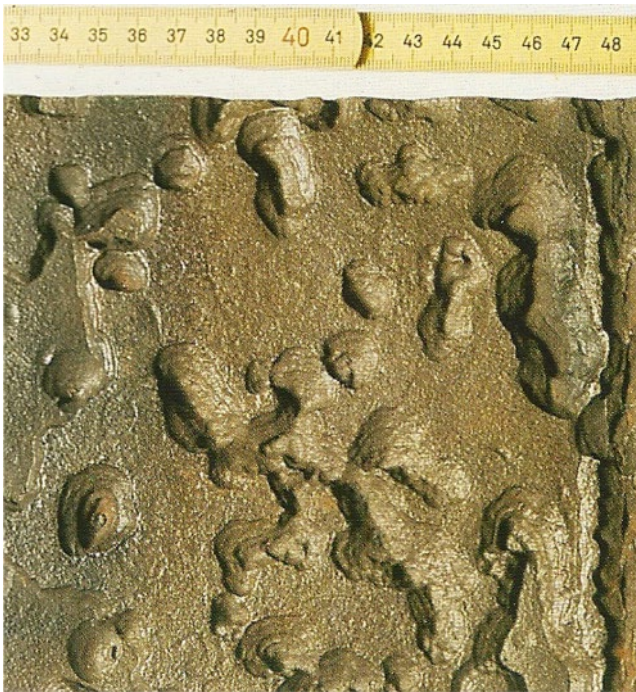
Figure 5.100 Mesa corrosion on carbon steel plate. Source: Bogaerts [82]. Reproduced with permission of NACE International.
