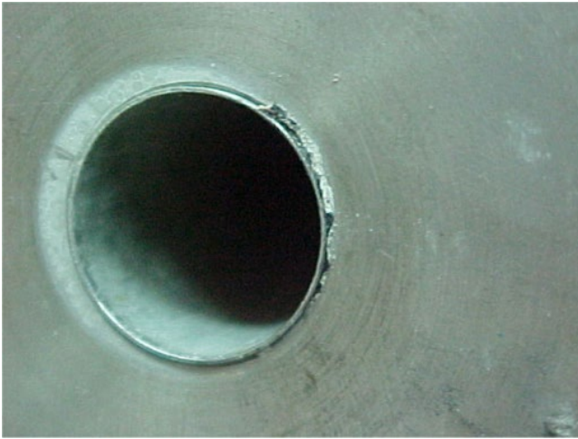
Figure 5.43 Crevice corrosion on a stainless steel heat exchanger [54]. Source: Reproduced with permission of John Wiley & Sons.
