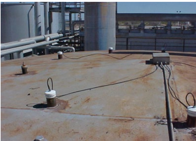
Figure 8.50 Impressed current cathodic protection anode lead wires on the top of a large AST.
