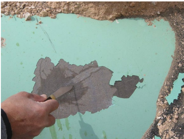
Figure 8.94 Underlying metal after nonadherent coating removed in the vicinity of the coating blister shown in Figure 8.93. Source: Photo courtesy R. Norsworthy, Polyguard Products, Inc.
