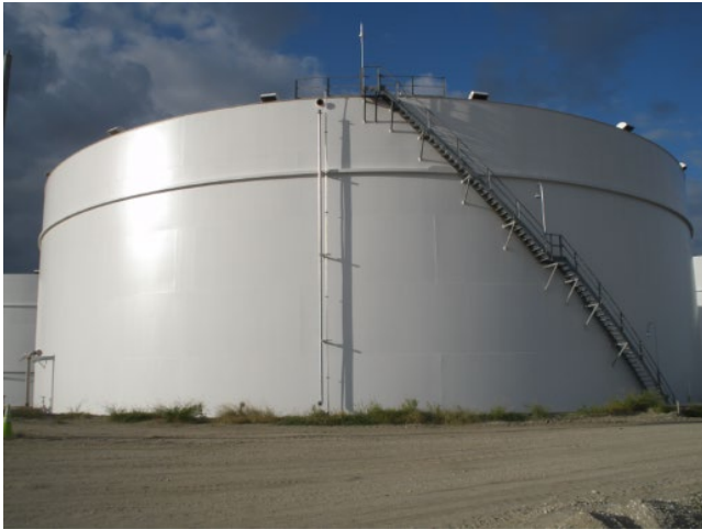
Figure 8.41 The painted exterior of the same aboveground storage tank shown with stripe coating in Figure 6.20.
