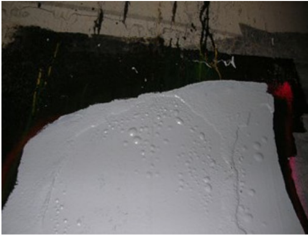
Figure 6.53 Blisters formed on light-colored repair coating due to improper surface cleaning. Source: Reproduced with permission of NACE International. Brodar presentation.
