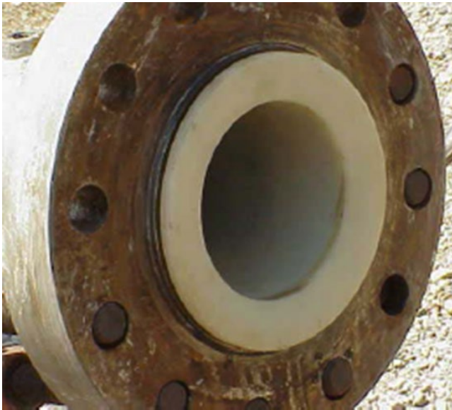
Figure 7.16 Flange near damage shown in Figure 7.15.
