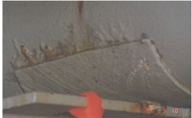
Figure 5.46 CUPS due to contoured fiberglass pads producing crevices if improperly sealed. Source: Reproduced with permission from Deepwater Corrosion Services Inc. [56].
