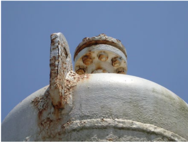
Figure 6.23 Corrosion on a complicated geometry structure needing grinding and smoothing plus stripe coating after surface preparation.
