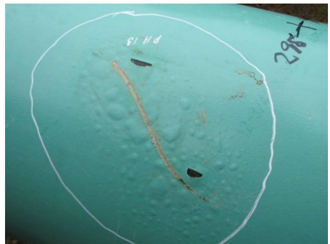
Figure 6.45 Coating blisters forming around scratches on a pipeline coating. Source: Photo courtesy R. Norsworthy, Polyguard Products, Inc.
