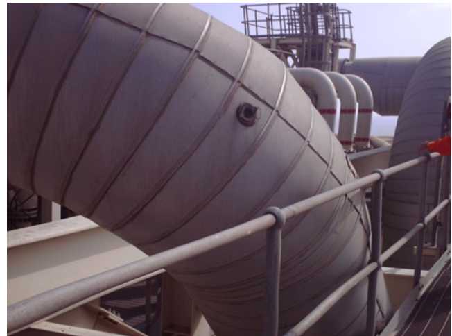
Figure 7.3 Ultrasonic inspection port installed near a walkway instead of a location likely to produce useful data.
