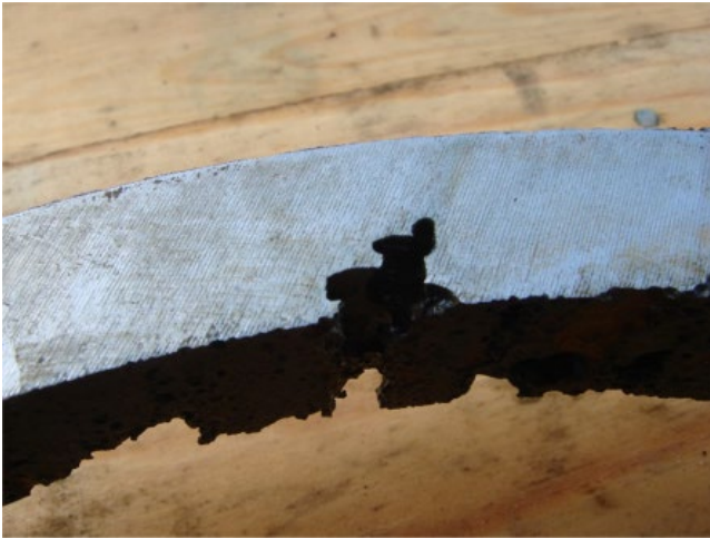
Figure 5.32 Internal corrosion pits formed on carbon steel pipe on an offshore platform.
