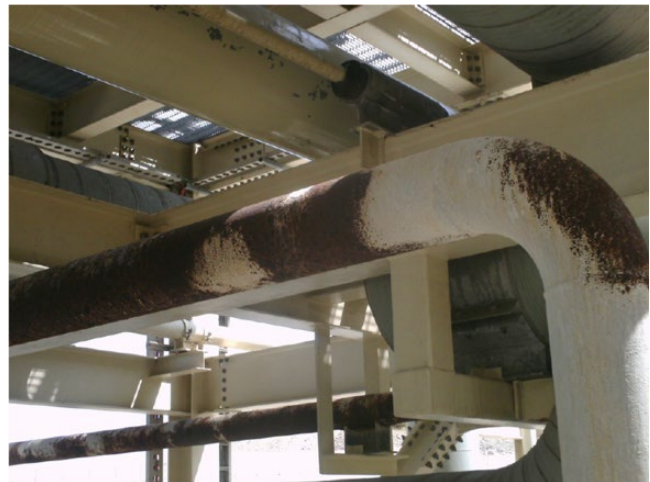
Figure 5.2 Localized general corrosion caused by fog condensation dripping from overhead equipment onto process piping.
