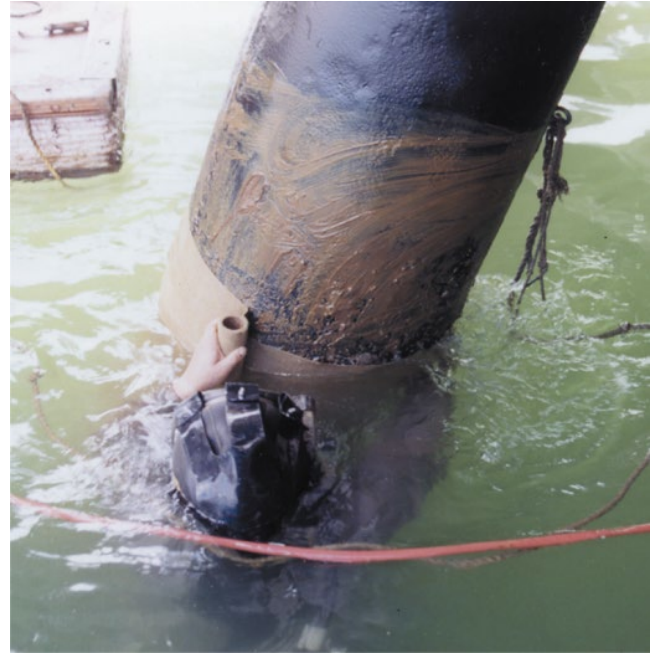
Figure 6.33 Repair wrap being installed on the tidal and splash zone portions of a marine piling. Source: Photo Courtesy Denso, Inc.
