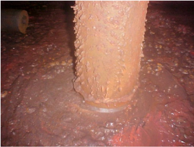
Figure 8.48 Corrosion on a vertical column at the bottom of a large AST.
