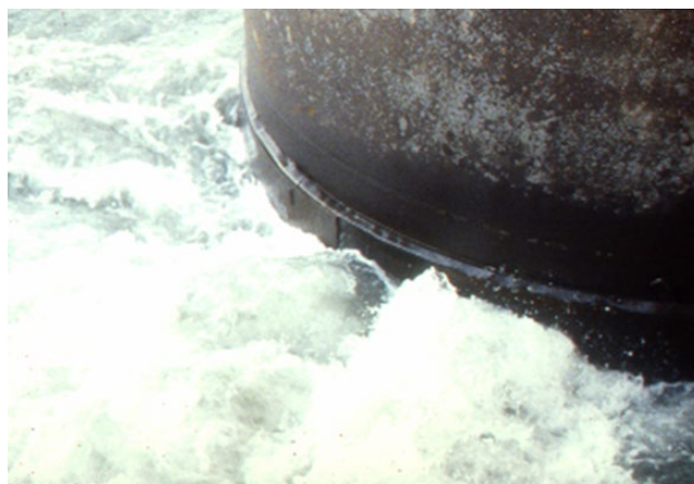
Figure 1.4 Offshore platform leg in Cook Inlet, Alaska. The extra metal for the corrosion allowance is submerged twice a day during high tides.
