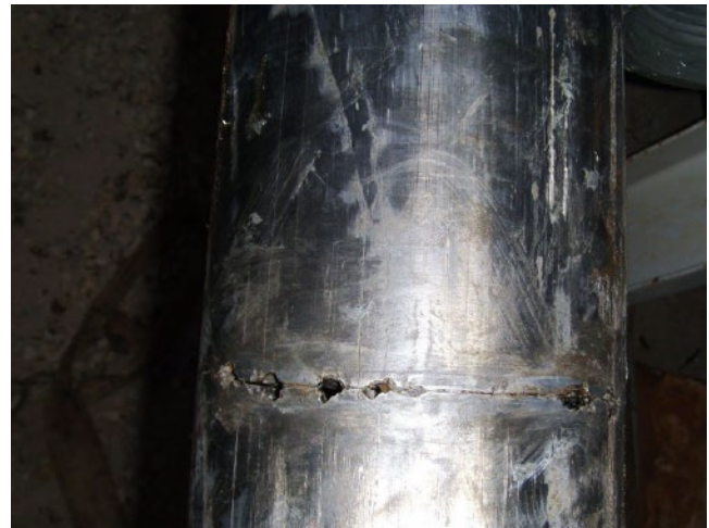
Figure 8.4 Drill pipe corrosion fatigue cracking and washout by drilling mud.
