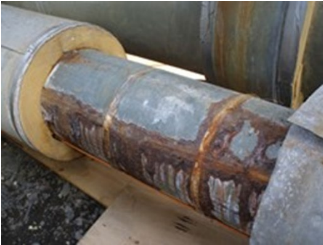
Figure 8.63 Corrosion underneath insulation on a crude oil piping system.
