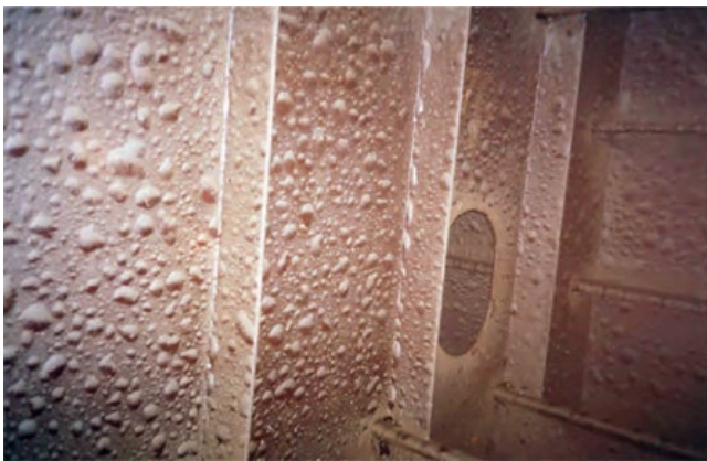
Figure 6.43 Extensive blistering on continuously wetted surfaces indicating inadequate surface preparation [69, 70]. Source: Reproduced with kind permission of Brendan Fitzsimons, FITZ-COATINGS Ltd.
