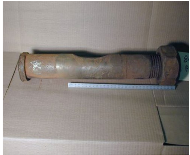
Figure 5.115 Fretting corrosion of a shackle pin from an FPSO mooring chain. Source: Photo courtesy Ammonite Corrosion Engineering, Calgary, AB, Canada.
