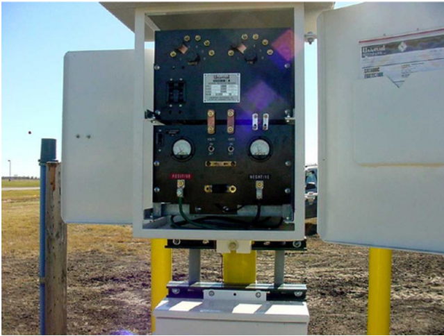
Figure 6.80 A typical cathodic protection rectifier used for onshore cathodic protection. Source: Photo courtesy NACE International.
