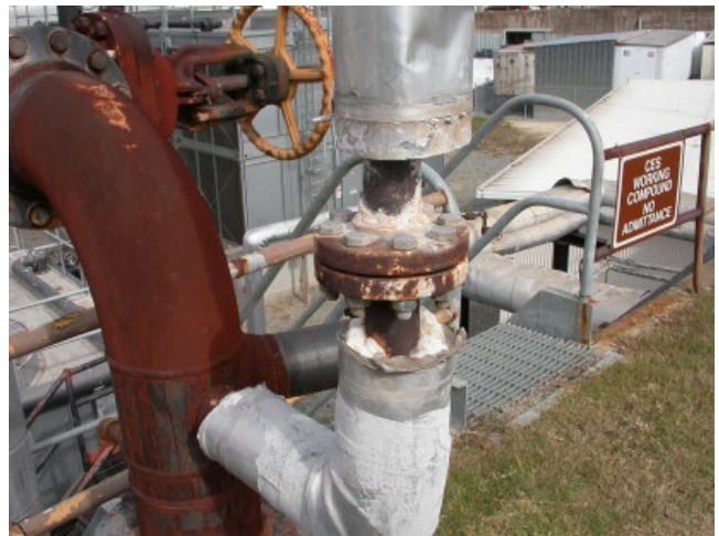
Figure 3.21 Insulation removed for maintenance and not replaced.
