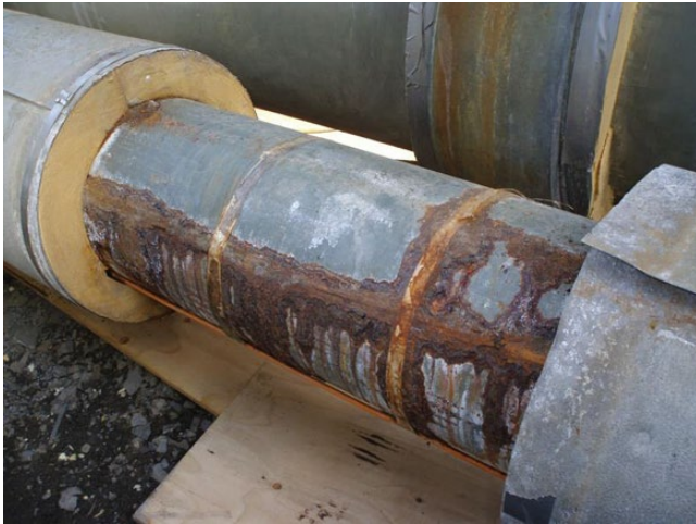
Figure 3.22 Missing protective coating near welds on insulated crude oil piping.
