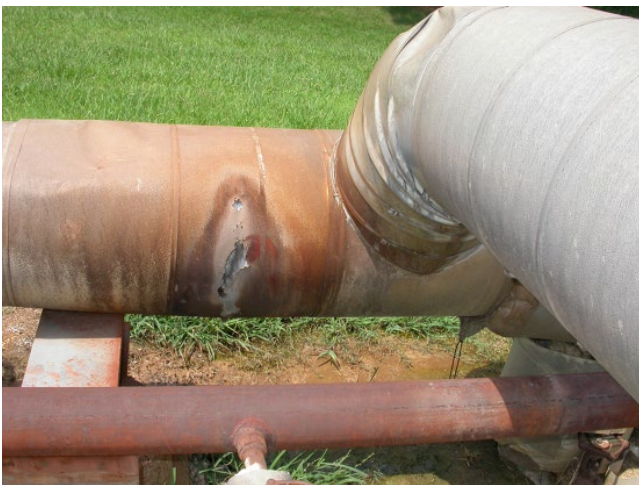
Figure 8.65 Aboveground insulated piping.
