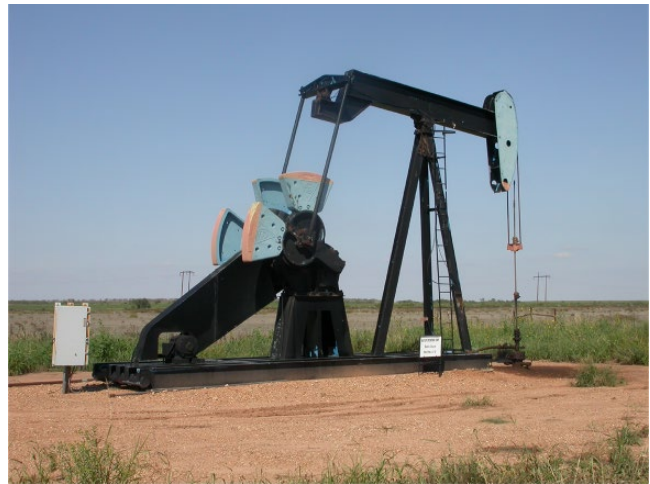
Figure 8.28 Topside of a beam pumping unit.
