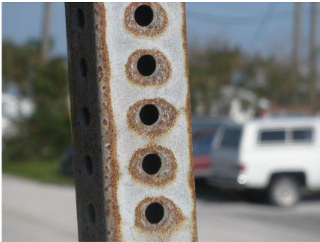
Figure 6.61 Corroded galvanized sign pole.
