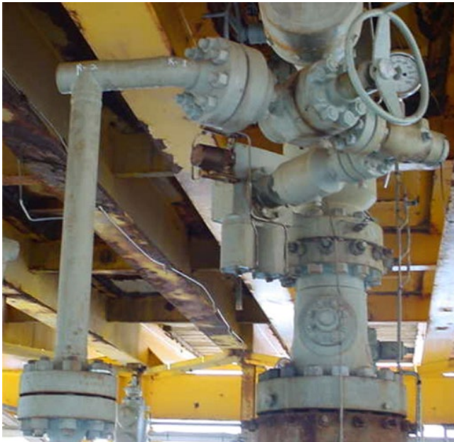
Figure 8.35 Christmas tree attached to a wellhead.
