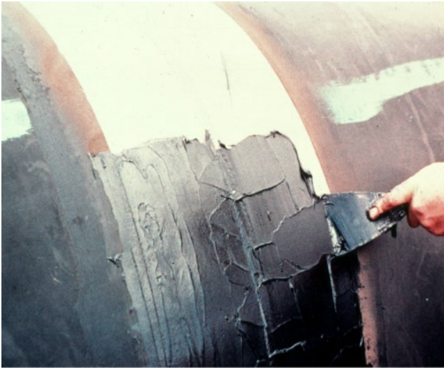
Figure 6.10 Trowel application of thick-film single coating of coal-tar urethane for field application at pipeline joints. Source: Courtesy of NACE International, reproduced with permission.
