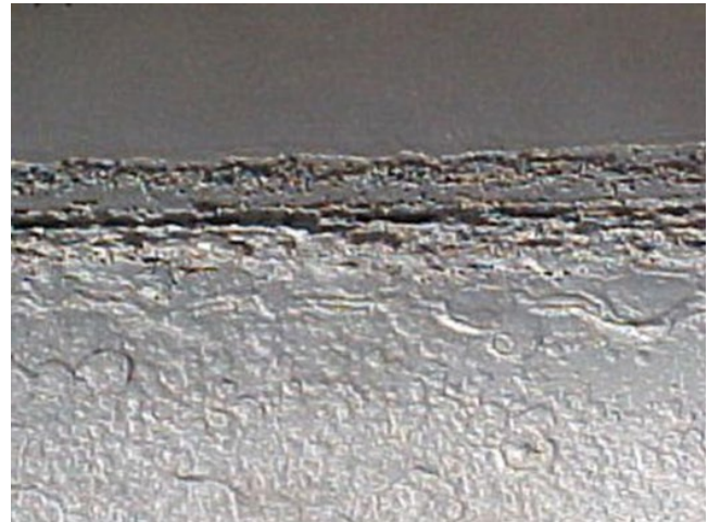
Figure 8.81 The interior of a natural gas pipeline showing the lack of corrosion in the gas phase and extensive pitting corrosion in the water and condensate phase.
