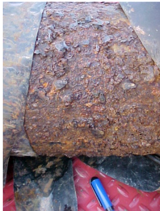
Figure 6.34 Pitting of underground pipeline where wrap was ineffective in preventing corrosion.
