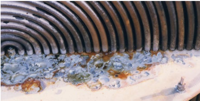
Figure 5.37 Pitting corrosion of an Alloy 825 (UNS N08825) heat exchanger baffle exposed to seawater [51]. Source: Courtesy of NACE International.
