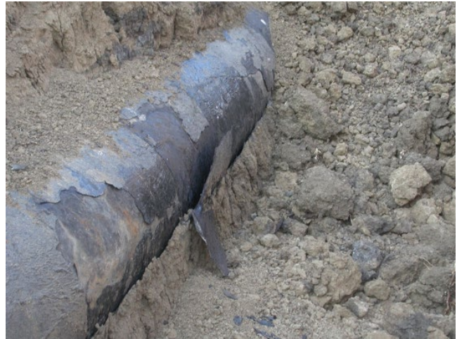
Figure 8.92 Disbonded pipeline coating.
