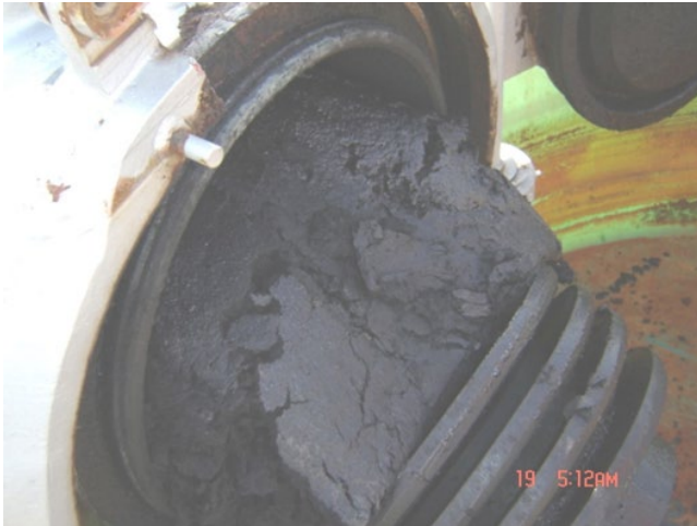
Figure 8.85 Black powder removed from a gas pipeline at a pig trap.
