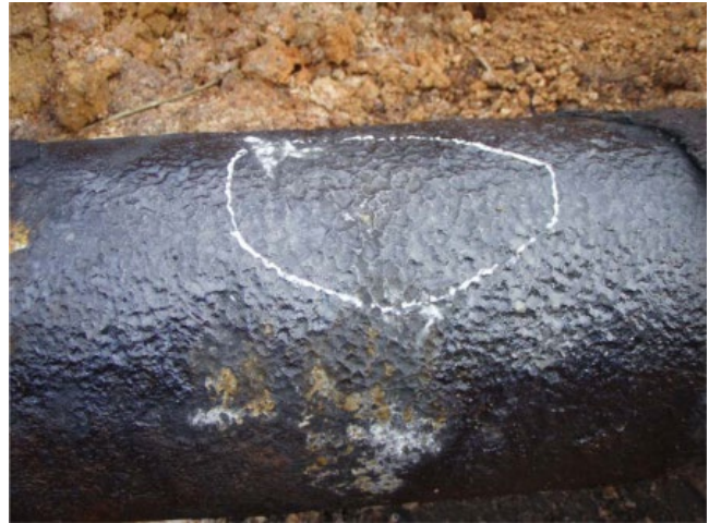
Figure 5.5 General attack of pipeline exterior beneath disbonded pipeline coating.
