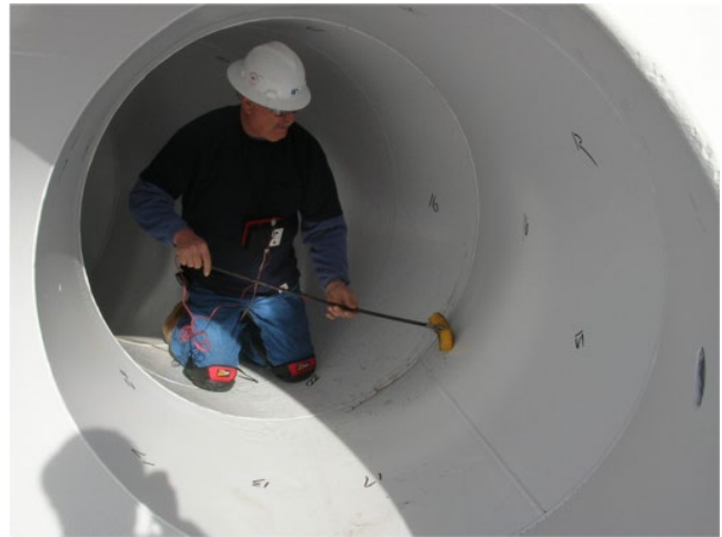
Figure 6.15 Electrical holiday testing in the interior of a large-diameter water pipe. Source: J. Brodar [25]. Reproduced with permission of NACE International.
