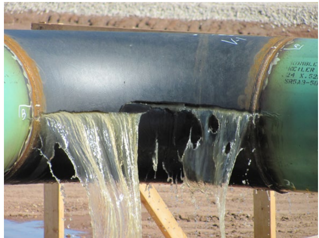
Figure 7.47 Crack and leak at seam weld during hydrostatic testing. Source: Photo courtesy J. Smart.
