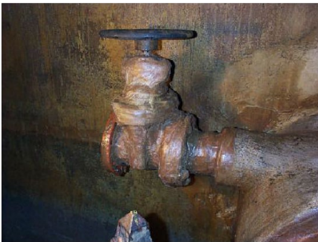
Figure 6.32 Waxed tape on a valve in a manhole.
