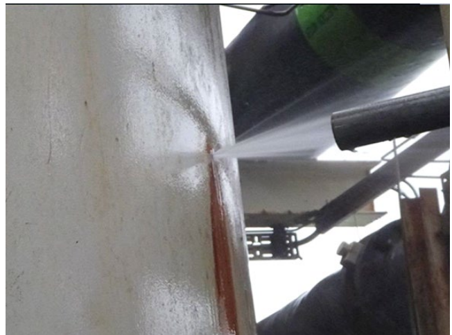
Figure 3.11 Leaking seawater filter vessel on an offshore platform due to waterline corrosion.
