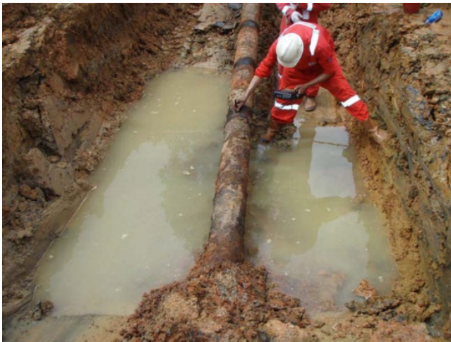
Figure 7.11 Ultrasonic inspection every meter at the 12 o'clock position on an exposed pipeline. Note the dark areas on the pipeline where dirt and debris have been removed so that good sensor contact can be maintained with the pipeline surface.
