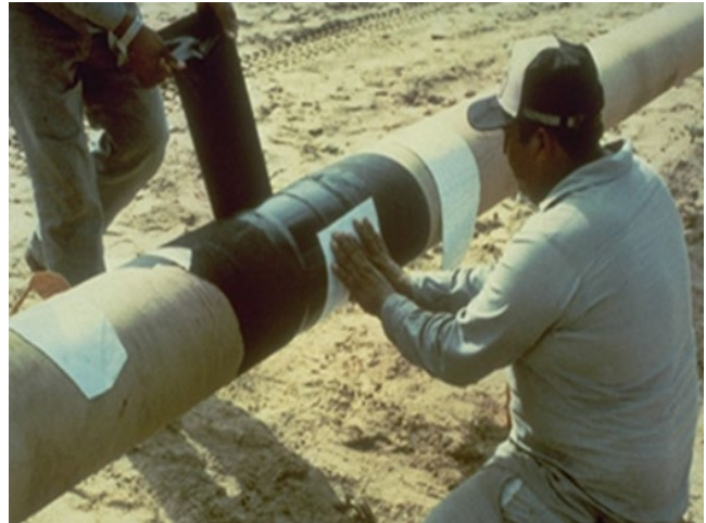
Figure 8.95 Application of a field-applied coating at a girth weld on a pipeline. Source: Photo courtesy NACE International.
