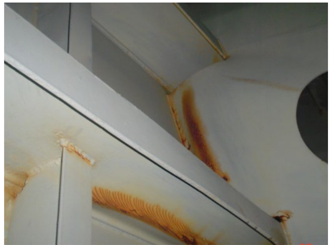
Figure 6.41 Cracking due to structural motion on the exterior wall of a vessel. Note the rust staining at locations where motion has occurred and at welds.
