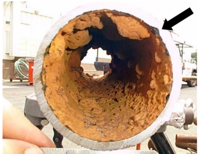
Figure 5.26 Pitting corrosion on carbon steel potable water pipe. Note the deepest pit at the two o'clock position on this 100 mm (4 in.) pipe.
