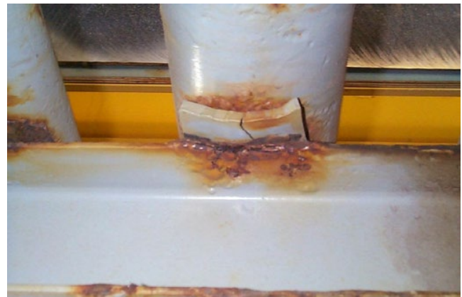
Figure 8.38 Corrosion of pipe at neoprene support gasket.
