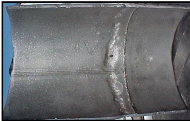
Figure 5.15 Heat-affected zone corrosion on carbon steel crude oil pipeline.
