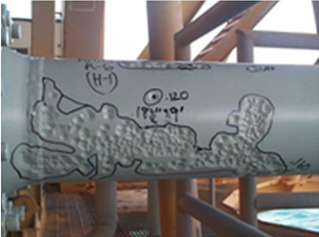
Figure 8.64 Localized pitting corrosion patterns underneath insulation on an offshore piping system.
