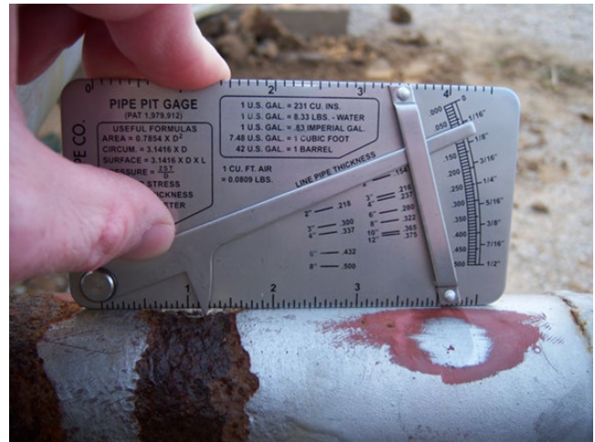
Figure 7.6 The use of a manual pit gage to measure the depth of external pitting on a pipeline.
