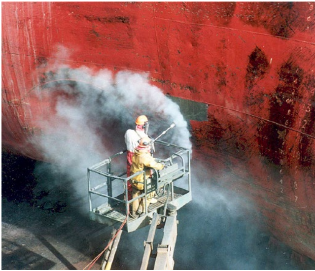
Figure 6.7 Water jetting surface preparation prior to recoating. Source: Photo courtesy of Hammelmann Corp., Dayton, Ohio, reproduced with permission.
