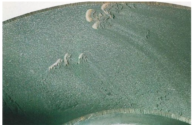
Figure 5.75 Erosion corrosion in a carbon steel steam pipe. Source: Bogaerts [82]. Reproduced with permission of NACE International.
