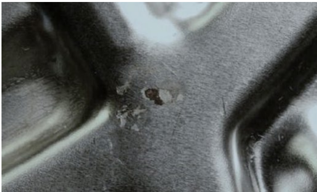
Figure 8.55 Crevice corrosion at contact point between two plates in a plate-frame heat exchanger [121]. Source: Reproduced with permission of NACE International.
