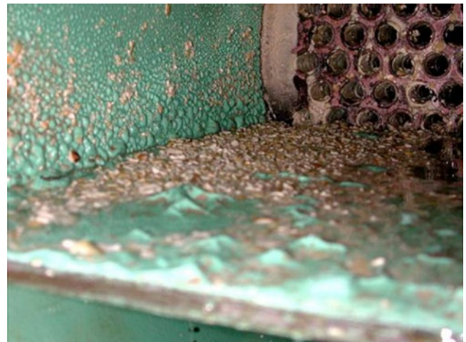
Figure 3.40 Scale formed inside a heat exchanger [24]. Source: Reproduced with permission of Springer.
