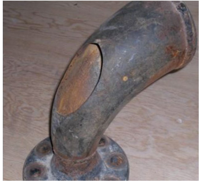
Figure 5.74 Erosion corrosion of an elbow in natural gas piping.
