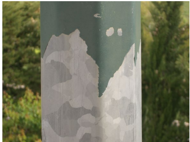
Figure 6.62 Disbonded coating on a galvanized pole.
