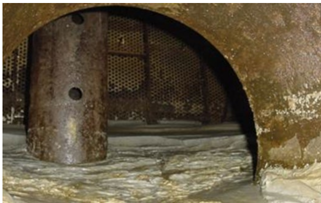
Figure 8.59 Sand accumulation in a free water knockout tank.
