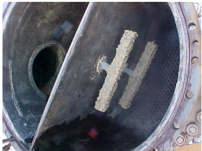
Figure 8.53 Magnesium anodes in the water-cooled header space on a gas cooler.
