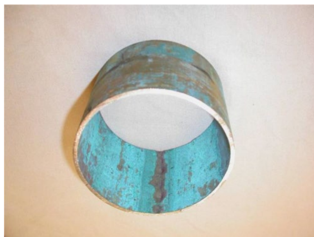
Figure 4.54 Underdeposit corrosion of 90–10 cupronickel tubing in offshore Gulf of Mexico firewater system.
