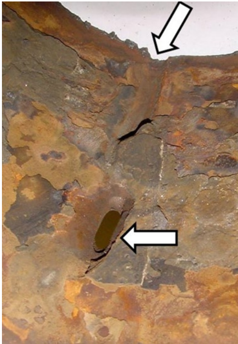
Figure 8.80 Six o'clock corrosion on a crude oil gathering line. Lower arrow shows pitting that produced leaking. Upper arrow highlights the profile of the pipeline.
