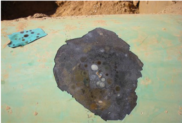
Figure 6.99 Whitish deposits underneath disbonded fusion-bonded epoxy coating. Source: Photo courtesy R. Norsworthy, Polyguard Products, Inc.
