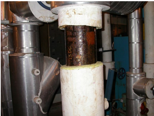
Figure 8.71 Condensation on the surface of an insulated chilled waterline where the insulation has not been replaced after repairs.
