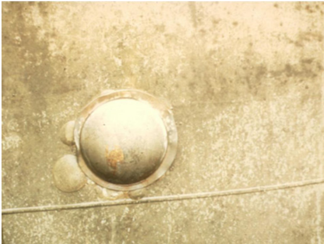
Figure 6.83 Coating disbonding caused by excessive current from a flush-mounted anode [135]. Source: Reproduced with permission of NACE International.
