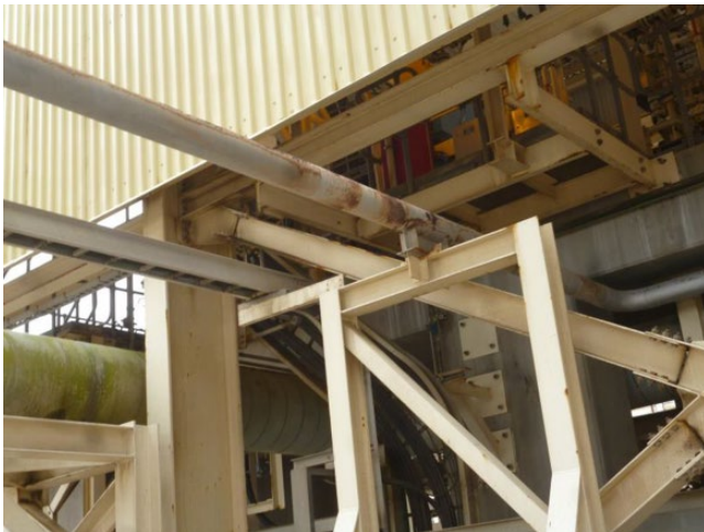
Figure 3.7 Localized atmospheric corrosion at the same facility shown in Figure 3.6.
