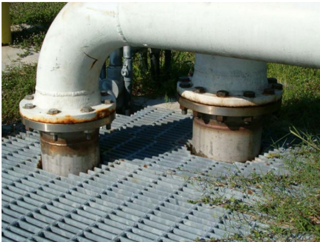
Figure 5.12 CRA fasteners on flange connecting carbon steel piping to CRA piping.
