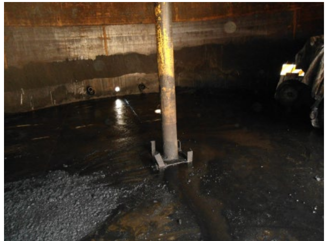
Figure 8.44 Bottom of crude oil AST showing solids buildup in the foreground and discoloration due to corrosion by water on the lower course of the steel wall in the background.
