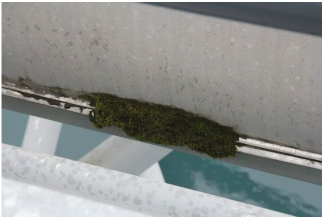
Figure 3.23 Moss growing at a seam on insulated piping. This moss indicates that excess moisture is leaking from within the protective jacketing.
