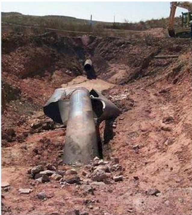
Figure 1.1 Natural gas pipeline rupture near Carlsbad, New Mexico, in 2000. Source: From Pipeline Accident Report [5].
