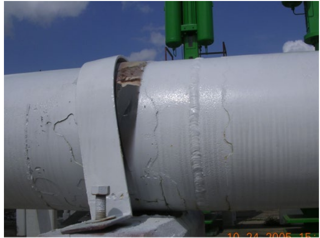
Figure 5.45 Crevice corrosion underneath the restraining strap on a pipeline. Source: Photo courtesy J. Byrd, Byrd Coating Consultants, Wellington, Florida, reproduced with permission.
