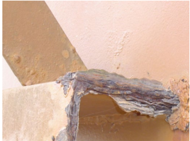
Figure 6.21 Flange on the exterior of an above-ground storage tank. All corrosion was ground away and the edges rounded before abrasive blasting and stripe coating.
