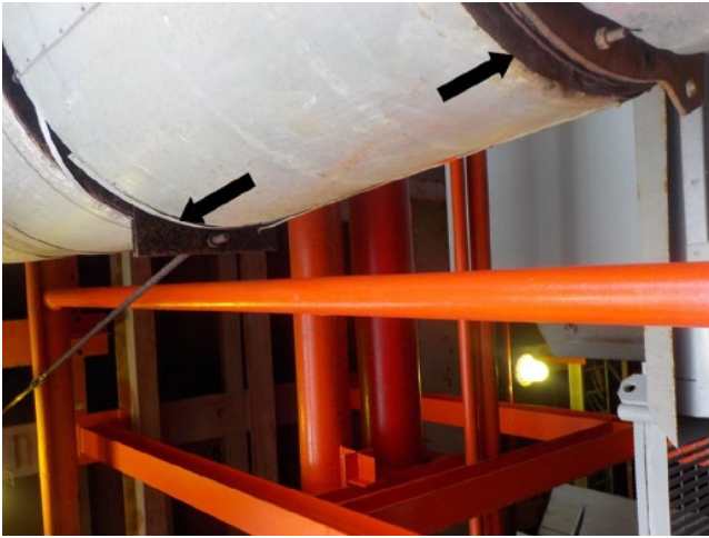
Figure 6.64 Corrosion of galvanized hardware around relatively uncorroded aluminum jacketing on an insulated offshore platform piping system. The arrows indicate the galvanized steel, which is exposed to a tropical marine atmosphere.
