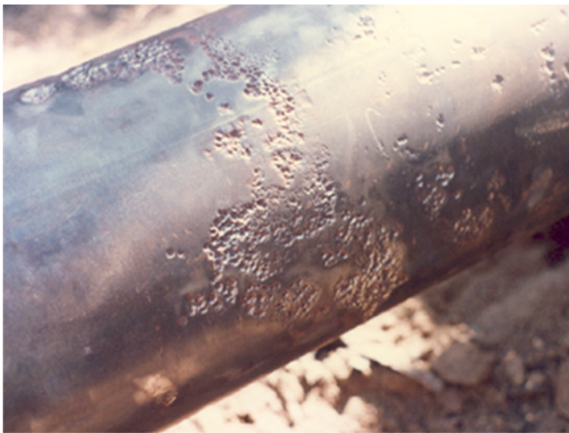
Figure 6.100 Pitting due to disbonded coating, which shielded cathodic protection current. Source: Photo courtesy R. Norsworthy, Polyguard Products, Inc.
