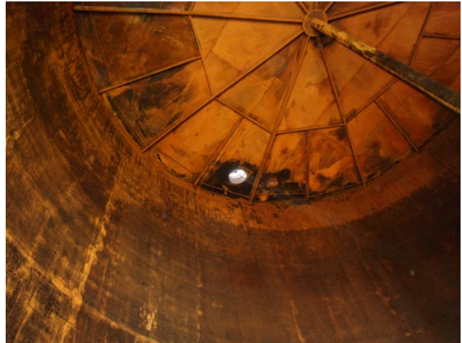
Figure 8.43 Corrosion on the interior ceiling of a crude oil AST.
