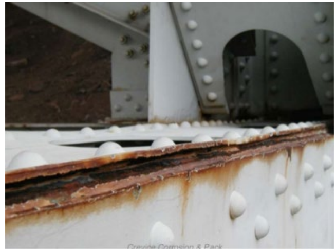
Figure 5.50 Distortion of structural steel caused by pack rust. Source: Reproduced with permission from Sabnis [59].
