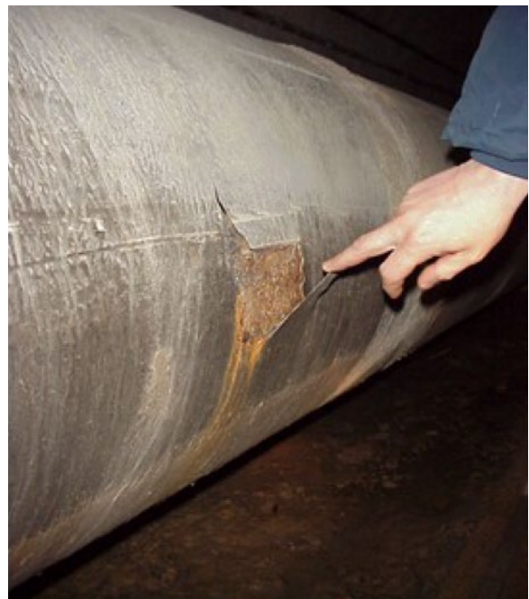
Figure 6.47 Protective coating lifting from the surface of a pipe due to corrosive undercutting. Source: Reproduced with kind permission of Brendon Fitzsimons, FITZ-COATINGS Ltd.
