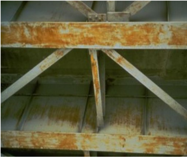
Figure 6.59 Pinpoint rusting. Source: Reproduced with permission of NACE International. NACE CIP 1–5.
