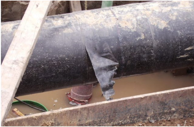
Figure 6.35 Low-build nonadhesive wrap coming loose from aboveground pipeline. Source: Photo courtesy Sandra Munoz, Corrosion y Proteccion, Cuernavaca, Mexico.
