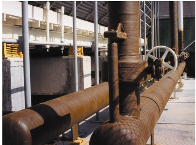
Figure 6.30 Petrolatum tape wrap on cooling tower piping. Source: Photo courtesy Denso North America Inc.
