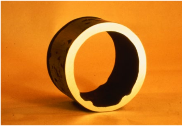
Figure 5.4 General corrosion along the bottom of a gas well flowline where acidic condensate thinned the bottom of this horizontal piping. It is obvious that the acidic water flowed at two different levels during the lifetime of this equipment. Source: Byars [9]. Reproduced with permission of NACE International.
