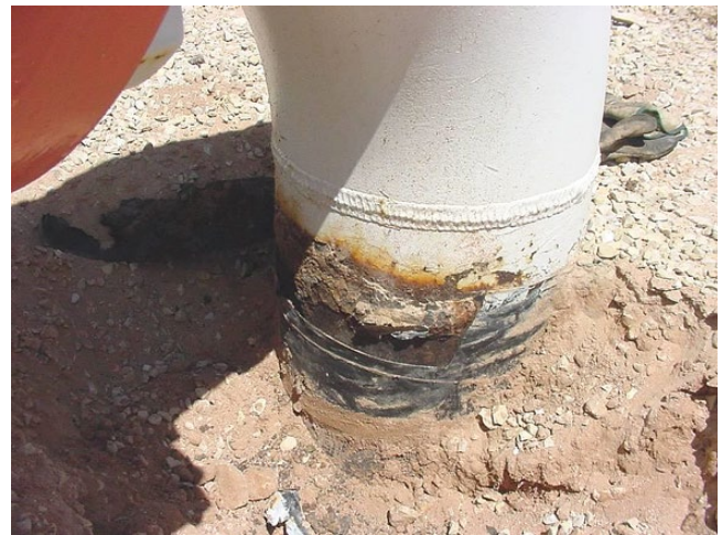
Figure 3.15 Corroded pipeline at the air-to-soil interface.
