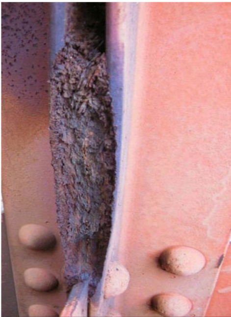
Figure 5.52 Close-up image of the metal distortion caused by pack rust. Source: Reproduced with permission from Sabnis [59].
