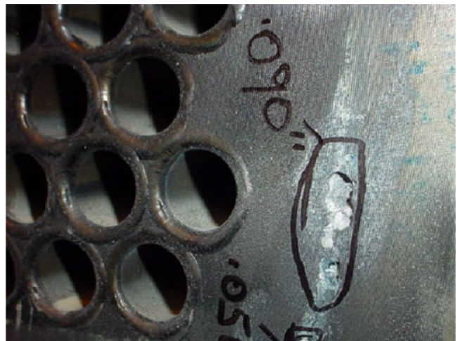
Figure 5.42 Crevice corrosion on a heat exchanger header plate.
