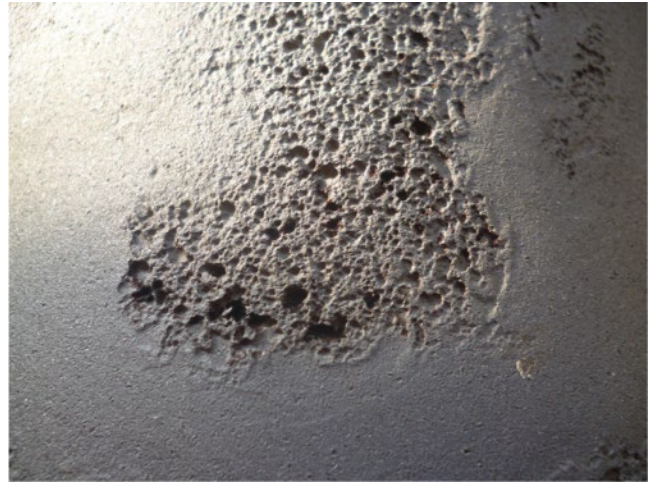
Figure 5.34 Colony of corrosion pits on stainless steel piping in a gas processing plant at a seaside location.
