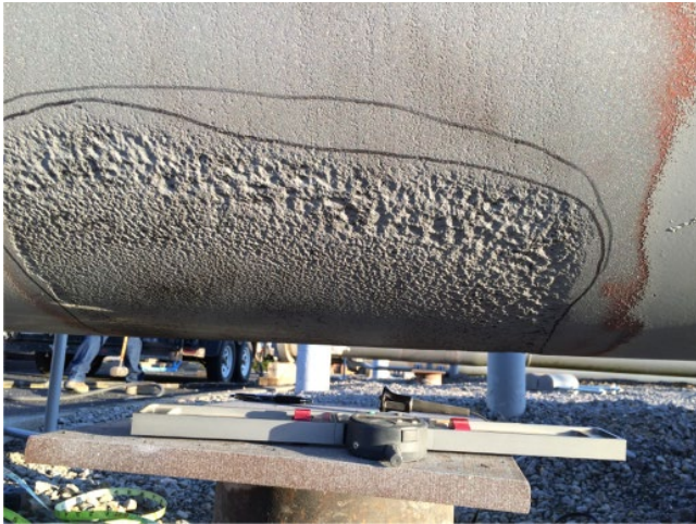
Figure 5.47 Pitting corrosion at a pipe support. Note how the pits are deeper away from the bottom (six o'clock) position.
