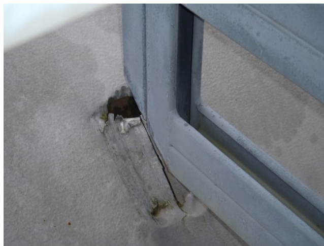
Figure 8.68 Penetration of exterior jacketing by support structure. Note how the original tight seal between the support and the jacketing has degraded over the years of service due to differences in the relative motion of the piping and the support.
