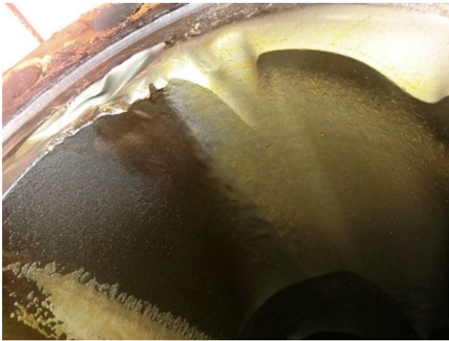
Figure 5.67 Smooth surfaces due to erosion corrosion on carbon steel piping downstream from a defective valve.
