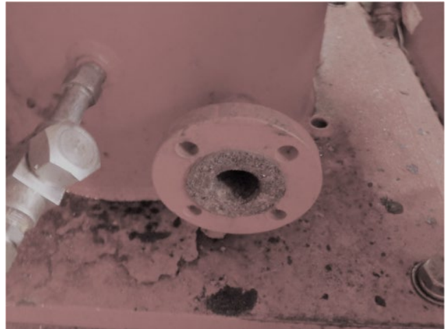
Figure 5.41 Crevice corrosion on a flange.
