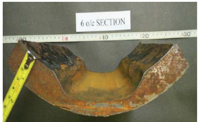
Figure 5.105 Severe channeling of a water injection pipeline. Source: Heidersbach and van Roodselaar [136]. Reproduced with permission of NACE International.
