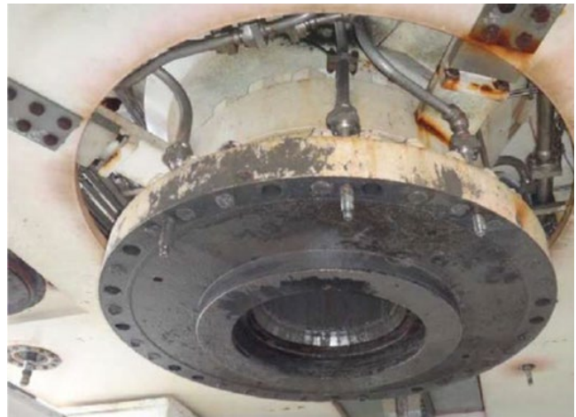
Figure 8.60 Upper half of a blowout preventer flange assembly where bolt failures led to system failure, with all 36 bolts failing under loading during service. These bolts, 51 mm (2 in.) in diameter, were made of UNS G43400 low-alloy steel, 34–38 HRC, and zinc electroplated [140–145].
