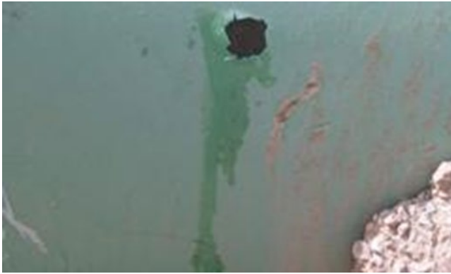
Figure 8.93 Blisters on fusion-bonded epoxy-coated gas transmission pipeline. Note the pH 12 water stains dripping from the broken blister. Source: Photo courtesy R. Norsworthy, Polyguard Products, Inc.
