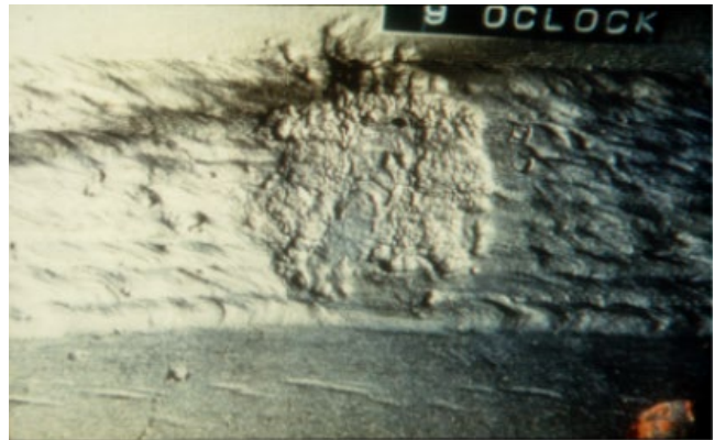
Figure 5.30 Corrosion pit on a weld of an offshore platform. The overlying marine growth and tubercules were mechanically removed to allow visual inspection using a remotely operated vehicle (ROV) with a television camera. Source: Smart [43]. Reproduced with permission of NACE International.
