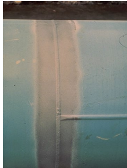
Figure 8.96 Field joint after blast cleaning. The factory-applied coating has been ground to provide a gradual transition for the subsequent field-applied coating. Source: Photo courtesy NACE International.
