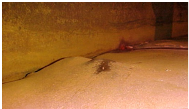
Figure 8.45 Ring bulging at outer wall of AST tank bottom. Source: Photo courtesy J. O'Hearn, Corpro, reproduced with permission.
