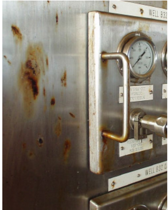
Figure 5.112 Contact corrosion on a control cabinet.
