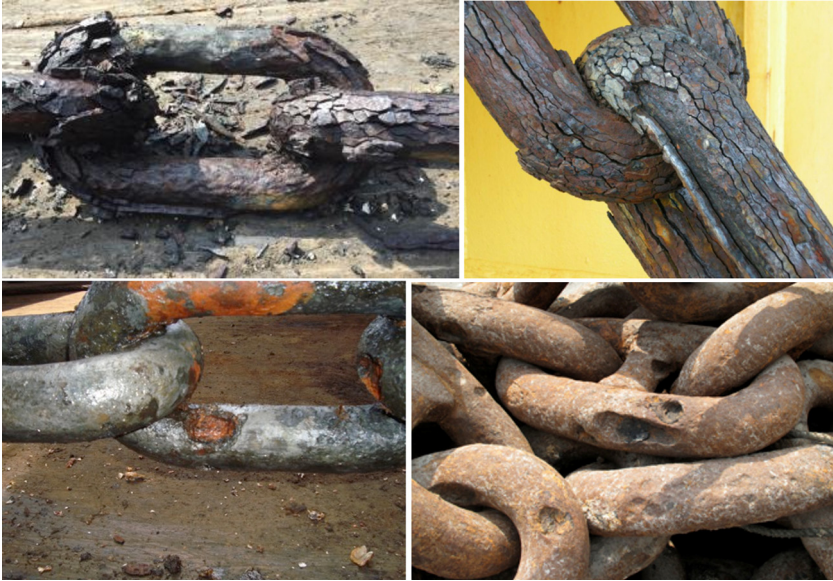
FIGURE 12.6 Chain with heavy general corrosion (top two); chain with large corrosion pits (bottom two) [7,8,12,13].
