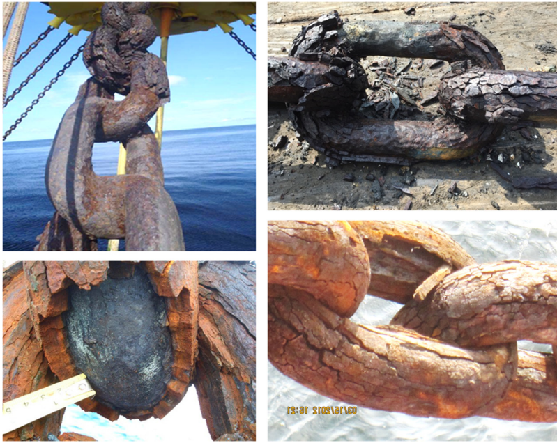
FIGURE 13.9 Examples of severe corrosion on chain in splash zone [37].
