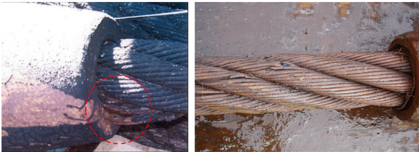
FIGURE 12.8 Broken wires at wire rope termination [14].
