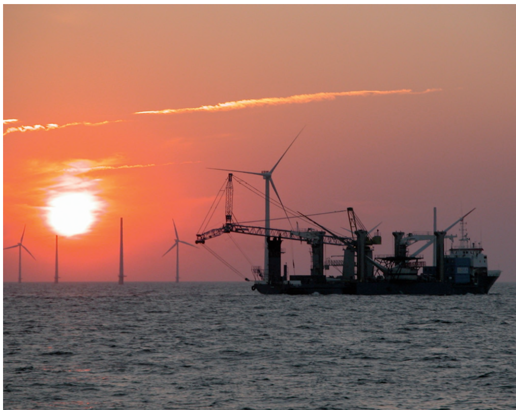
Fig 9.2.B A magnificent picture of a jack up vessel at work in an offshore wind farm. A similar vessel from A2SEA, the Sea Jack (formal Jumping Jack) can be lowered and lifted with fast acting winches. When the legs are lowered to the seabed, or the barge is being lifted, the lifting winches are applied with passive heave compensator systems to limit the force variations due to the heave of the barge. (Picture by Courtesy of A2SEA)
