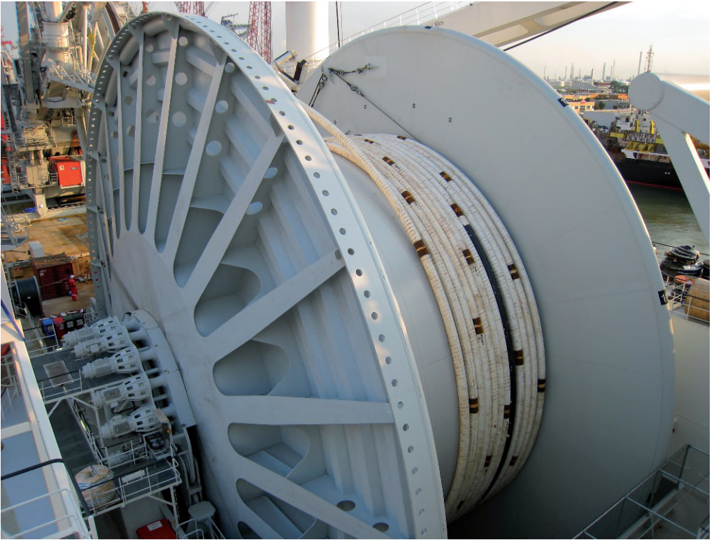
Fig 5.2.D. Electrical driven reel (AC induction motor with frequency drive) for the huge reel on the Seven Oceans of Subsea7 (Courtesy of Huisman)
