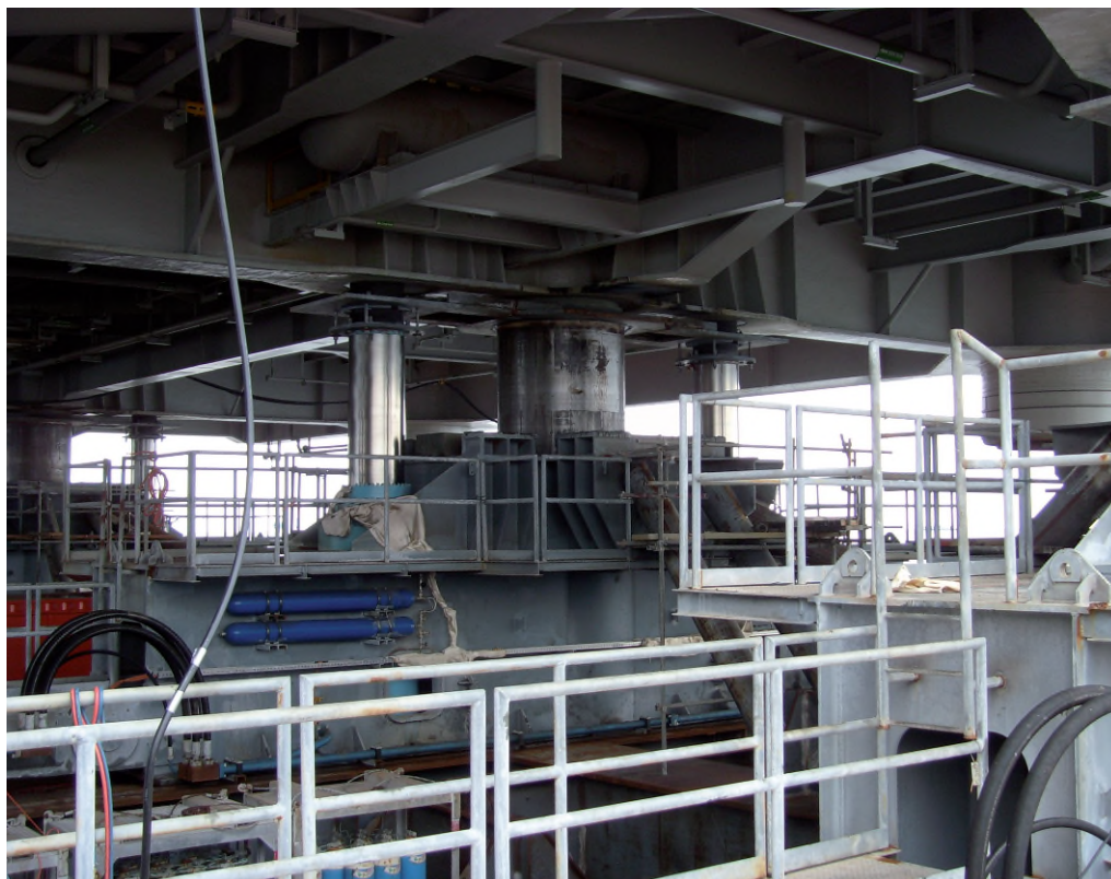
Fig 7.4.C Picture taken during the float over project from Heerema at the west coast of Nigeria. Eight of the shown jacks were used during the float over to lower the 12.300 mTon weighing topside onto its jacking structure. The cylinders were also lowered making use of large flow control valves. (Courtesy of Heerema)
