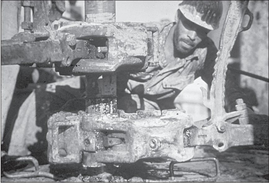
Plate 15–3. Tongs and spinning wrench being used on drillpipe. (Courtesy of API and Chevron.)
