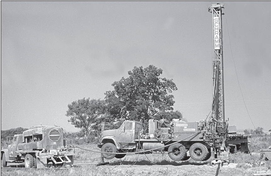
Plate 17-1. Truck-mounted air drilling rig. Note the smaller truck with an air compressor to the left. The blooie line is pointing out from the bottom of the drilling rig.
