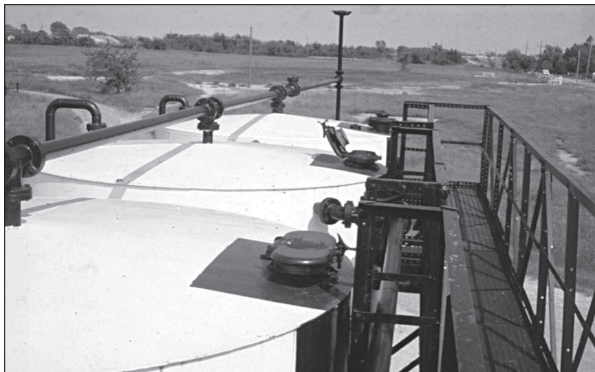
Plate 20-3. Top of stock tanks showing open and closed thief hatches and catwalk
