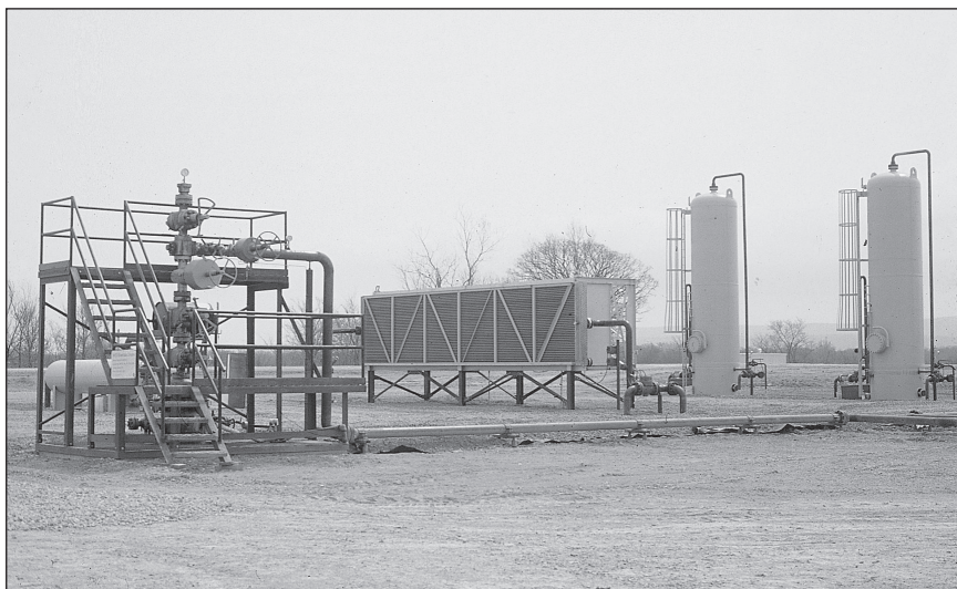
Plate 20–1. Christmas tree and gas-conditioning equipment
