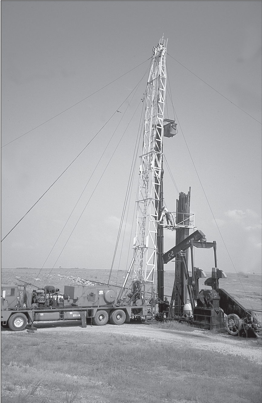
Plate 22–2. Well service unit with a structural mast that is pulling tubing. Note the tubing platform (lower) and rod basket (higher).
