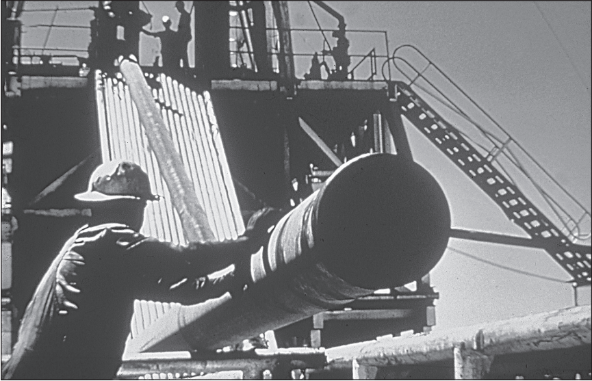
Plate 19–2. Casing being run up the pipe ramp onto the drill floor. (Courtesy of API.)
