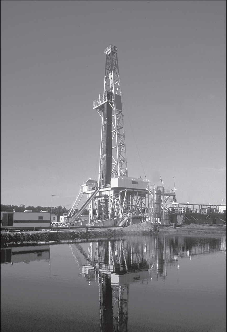
Plate 14-2. Wildcat well being drilled by a modern rotary drilling rig. (Courtesy of Parker Drilling.)
