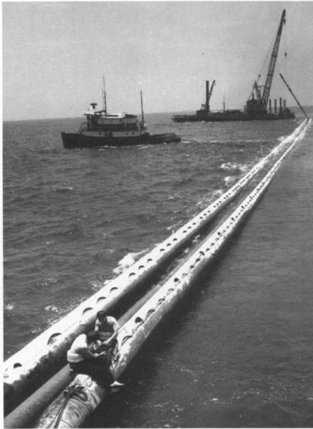
Wiring up the M-211 's 728-foot stinger to lay pipe for Shell's Marlin system
