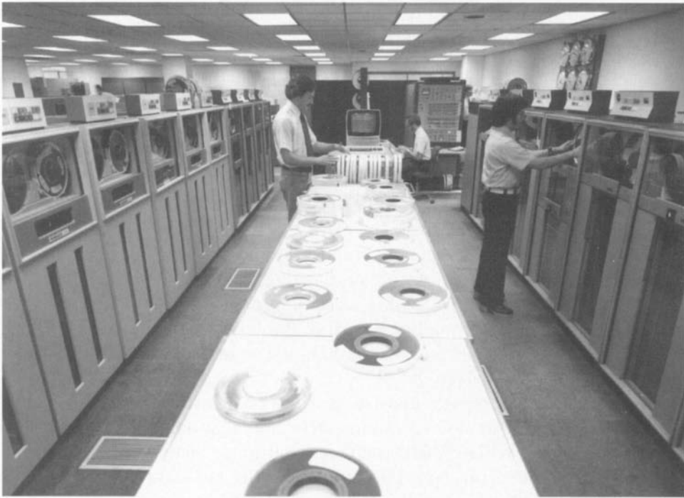
Computer room at Clinton Drive
