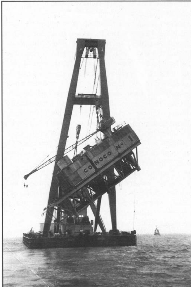
Broken A-frame with Conoco deck. Photo courtesy of Dirk Blanken
