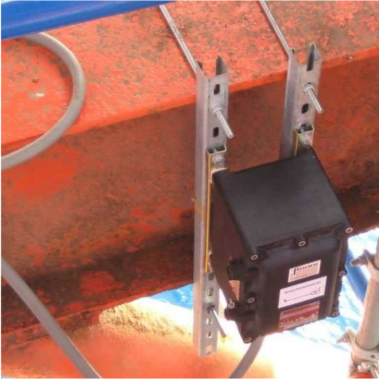
FIGURE 7.32 Vibration monitoring attached to the deck beam.
