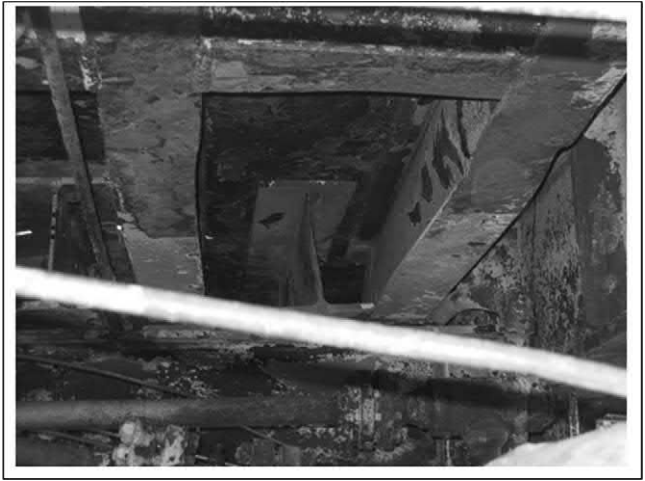
FIGURE 7.11 Fire-related deformation of the main and secondary beams for the deck.
