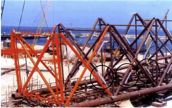
FIGURE 6.8 Locations of the anodes on the jacket during construction.
