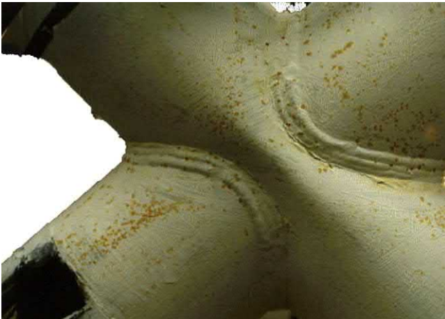
FIGURE 3.36 Buckling of the tubular joint.
