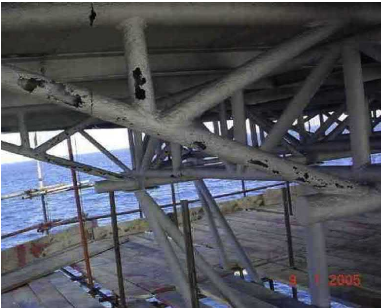
FIGURE 7.30 Severe corrosion of helideck main truss.
