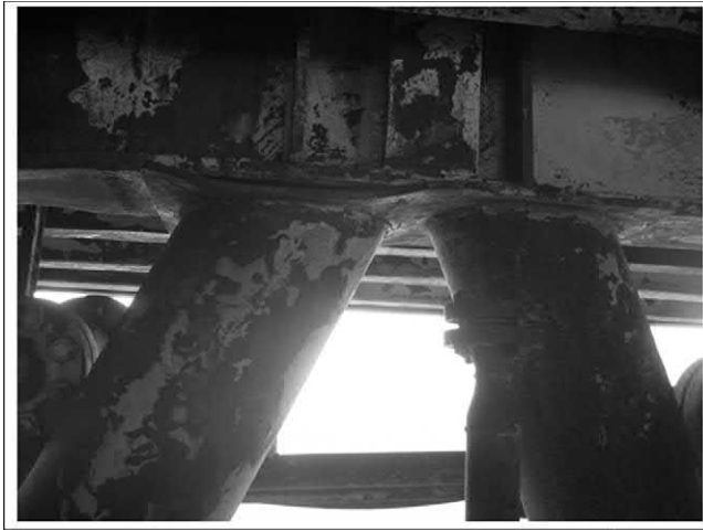
FIGURE 7.10 Fire-related effects on the main truss.
