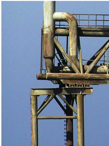
Figure 7.73 Flare bridge support.
