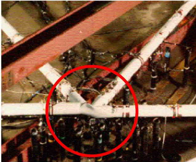
Figure 3.34 Failure in the K joint.
