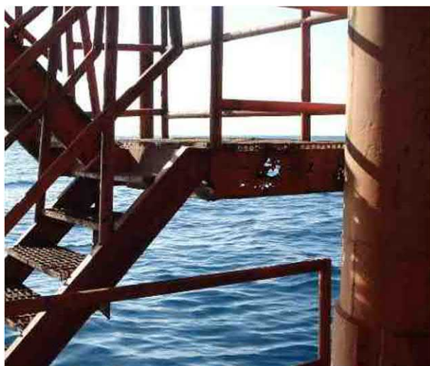
Figure 7.39 Severe corrosion damage to the stair.
