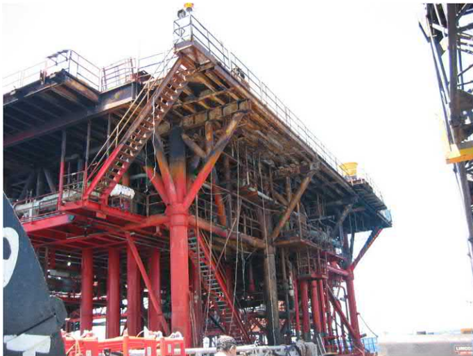
Figure 7.9 The fire on the main deck.
