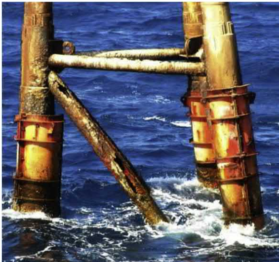
Figure 7.69 Loosening the clamp and corroded member.
