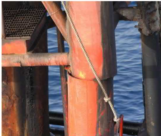
Figure 7.18 Failure on the leg.
