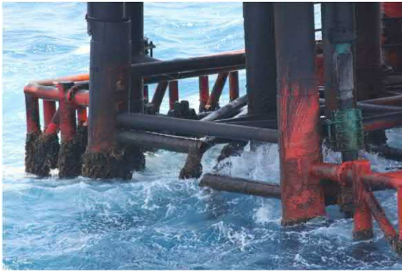
Figure 7.17 Failure on the bracing member.
