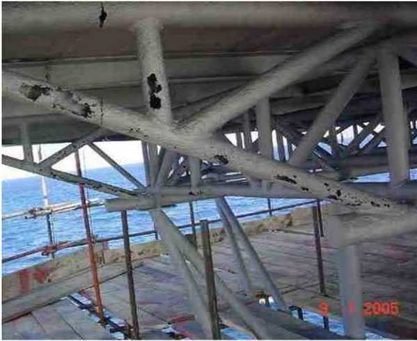
Figure 7.40 Severe corrosion to the helideck main truss.
