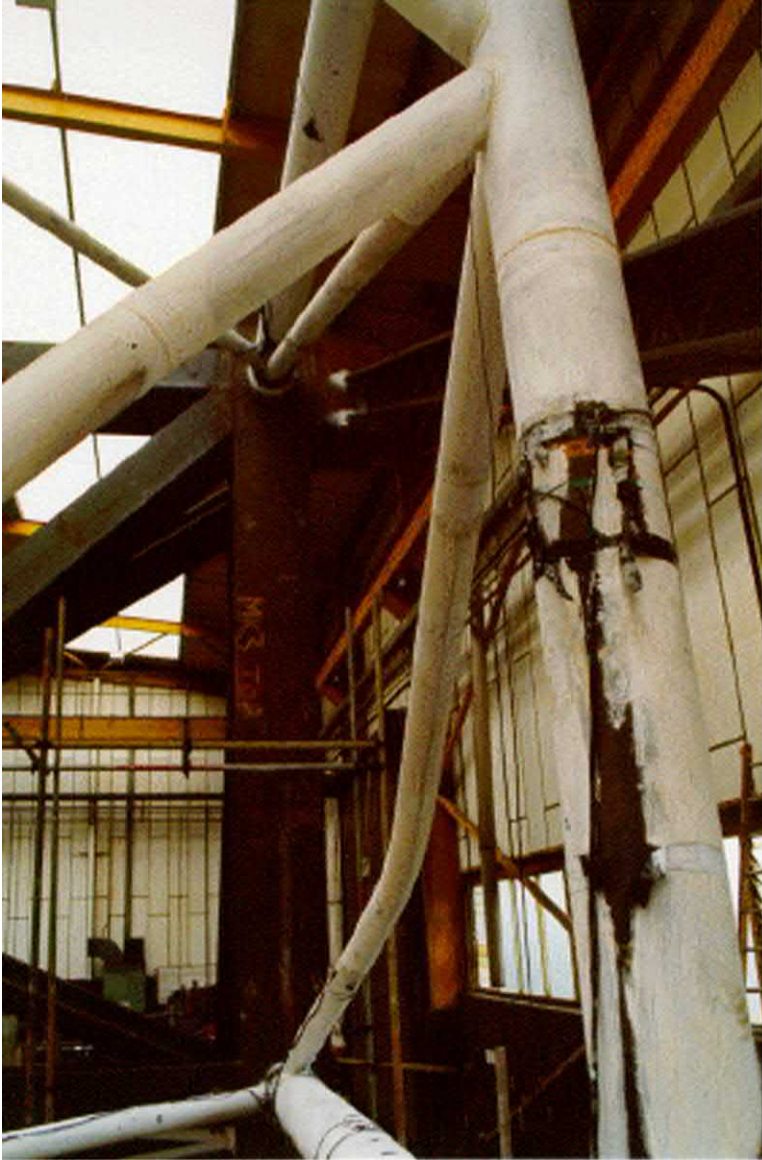
Figure 3.10 Buckling in the member for K bracing.
