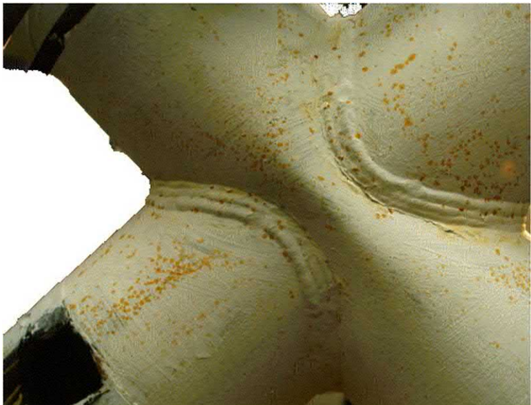
Figure 3.36 Buckling for the tubular joint.
