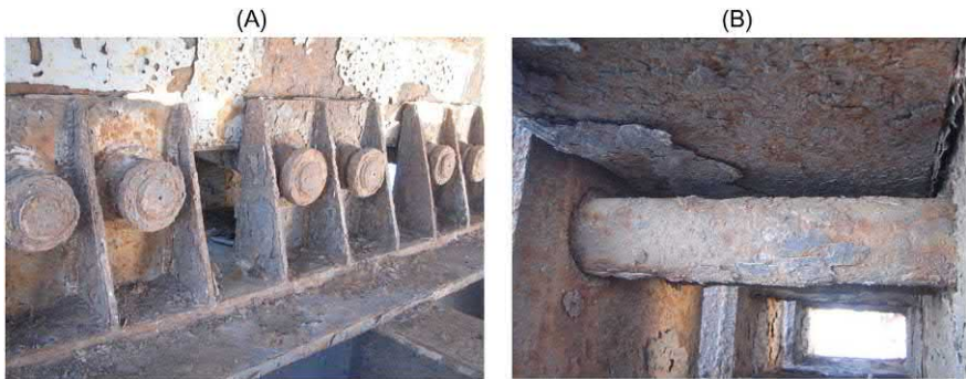
Figure 7.72 (A) Corrosion of bearing. (B) Corrosion of the bearing stud.
