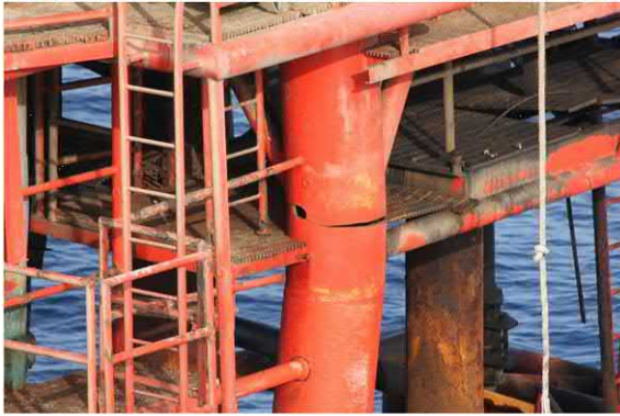
Figure 7.19 Shear cracks on the leg with rotation.
