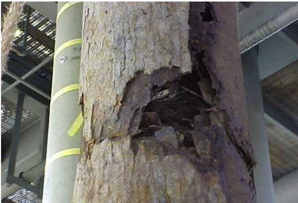
Figure 7.59 Severely corroded conductor.
