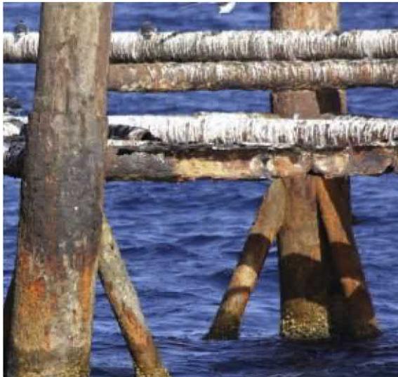
Figure 7.67 Corrosion in horizontal bracing.
