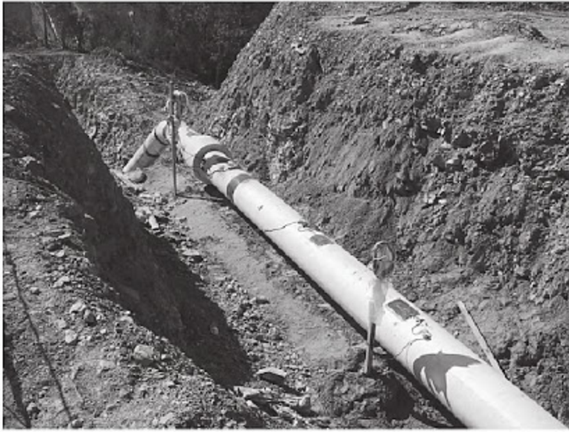
Electrodes used to monitor pipe potential
