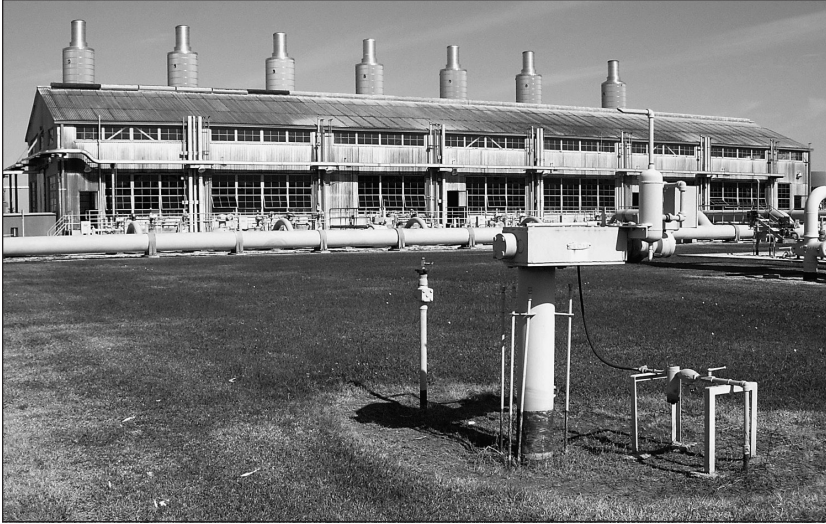
Fig. 9–5. Origination gas compressor station ( Source: Miesner and Leffler; photograph courtesy of Williams Gas Pipeline )
