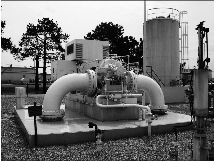
Fig. 9-6. Electric motor driving a centrifugal pump ( Source: Miesner and Leffler )
