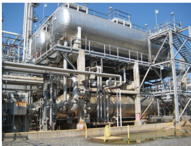
Figure 10.10 Photograph of an Alkylation unit (Source:www.phxequip.com/Multimedia/images/plant/original/refinery-alkylation-unit-390.jpg. All rights reserved.).
