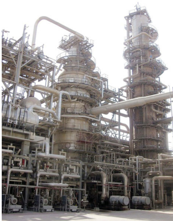
Figure 6.7 A photograph of the mild vacuum column, crude distillation tower with associated pumps, accumulators and piping.
