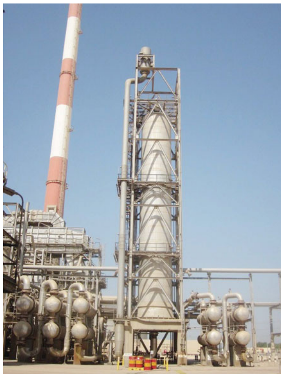
Figure 7.40 Heavy gas oil hydrodesulfurizer reactor with feed/effluent shell and tube heat exchangers.
