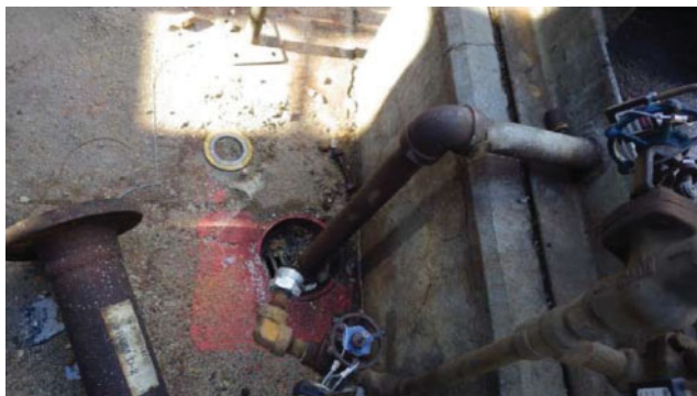
Figure 10.21 Typical pump drain to Oil Water Sewer (OWS) (Source: csb.gov).
