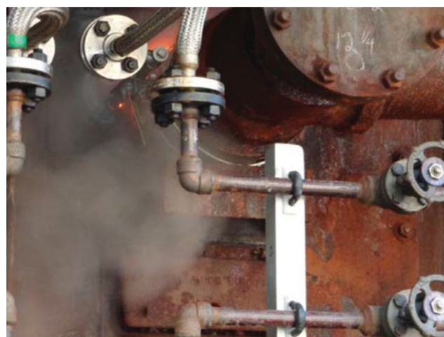
Figure 10.20 Burner on furnace (Source: csb.gov).
