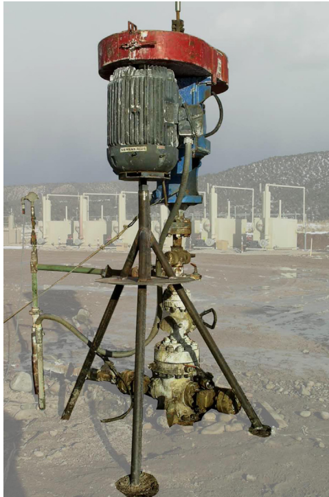
Figure 3.36 PCP support system.
