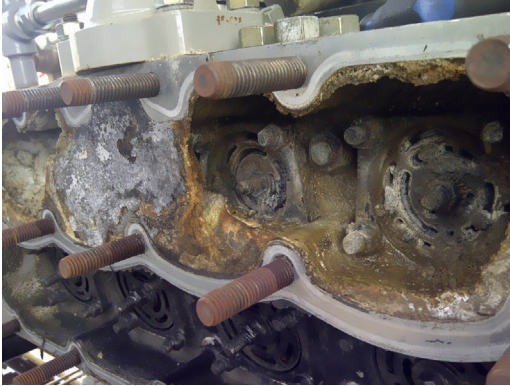
Figure 3.7 Salted reciprocating compressor valves. Source: Personal collection of Dejan Ivanovich.
