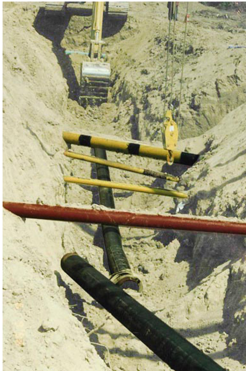
Figure 6.6 Foreign pipe crossing.
