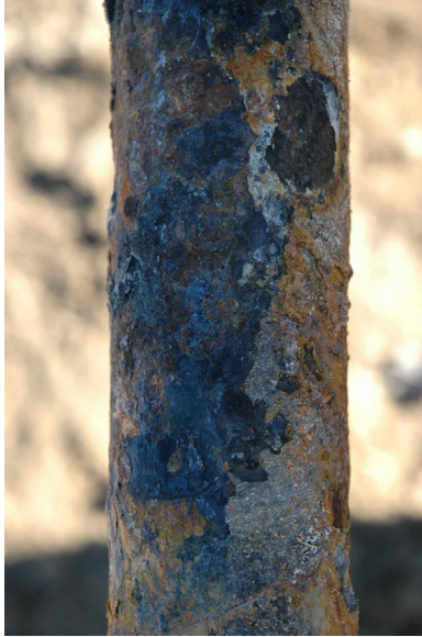
Figure 4.13 External galvanic corrosion.
