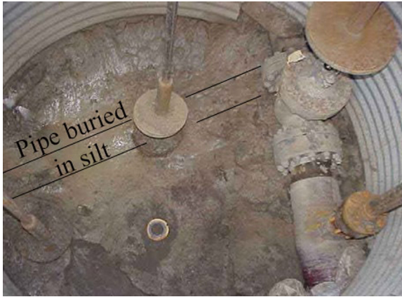
Figure 6.26 Valve can filled with silt.
