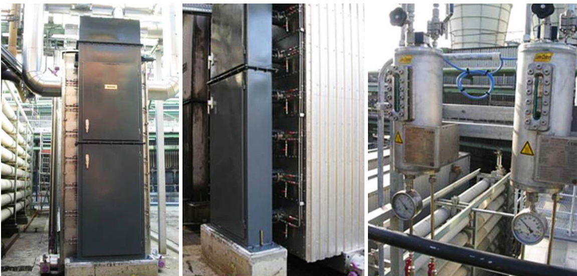
Fig. 33.41 Two end views of installed SSE and one top view above the SSE (long tubes near the bottom of the picture). (Photo courtesy of BORSIG)
