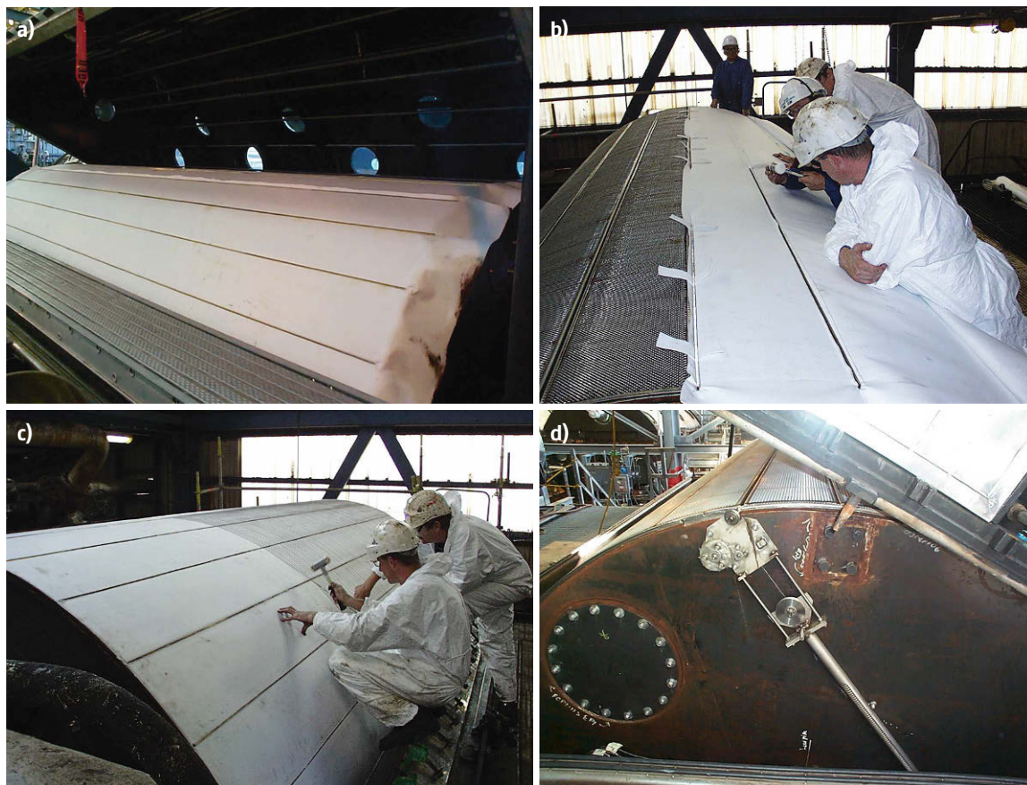
Fig. 33.50a–d Filter cloth installation. (a) Caulking bars hammered into caulking bar groove. (b) Removal of excess cloth. A small cloth strip is used in all grooves that do not have cloth overlap to provide tight fit. (c) Technicians tamp down the caulking bar as the wire is wound onto the drum. (d) Wire tension take up device. (Photos by B.E. Beasley, courtesy of ExxonMobil Process Research)
