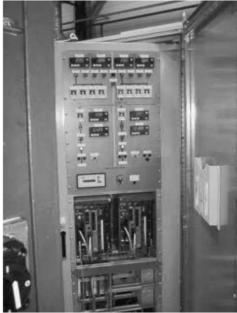
Figure 7.10 Electrical Power Unit (EPU).
