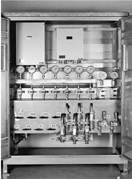
Figure 3-2 Topside Umbilical Termination Assembly (TUTA) [1].
