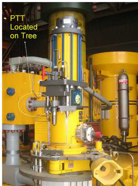
Figure 24-25 PTT Located on a Subsea Xmas Tree.
