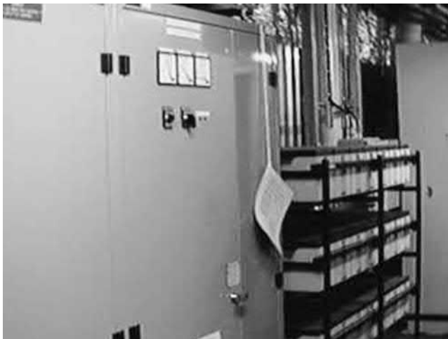
Figure 8-5 UPS and Battery Rack.
