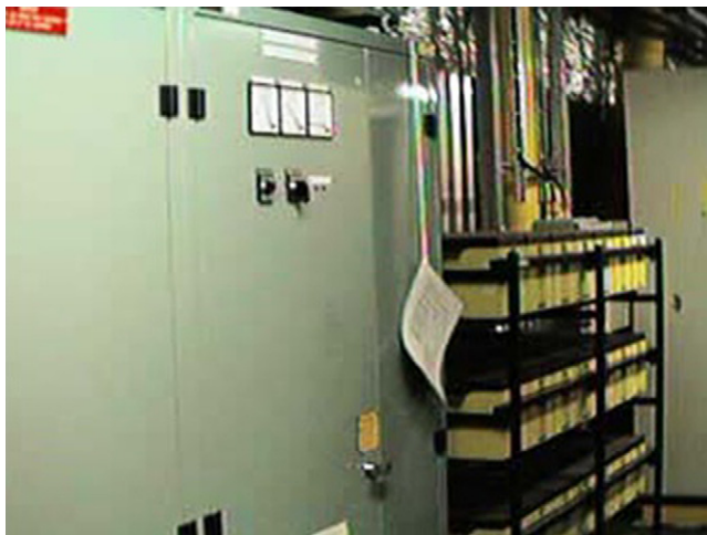
Figure 8-5 UPS and Battery Rack
