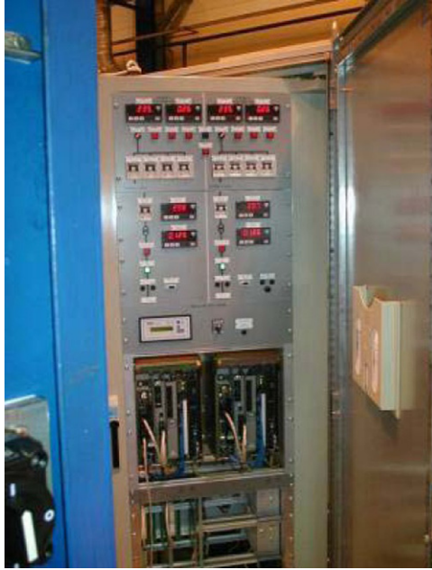
Figure 7-10 Electrical Power Unit (EPU)
