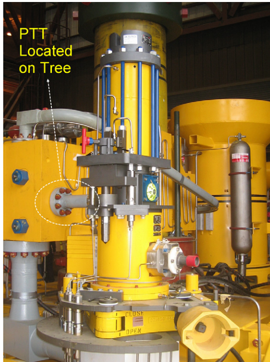
Figure 22-38 PTT Located on a Subsea Xmas Tree
