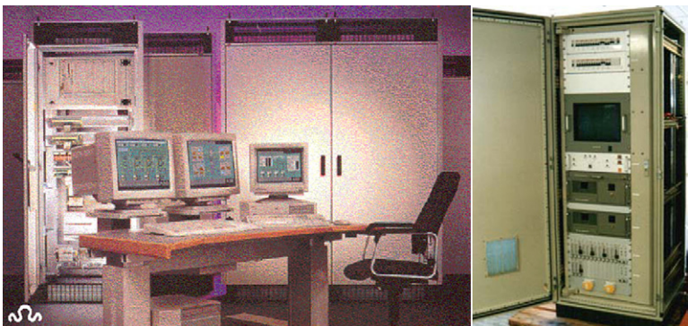
Figure 7-8 Mater Control Station (MCS)
