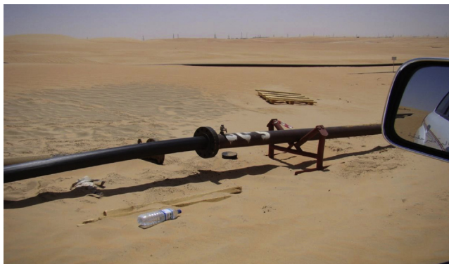
Figure 5.2 Insertion of high density polyethylene internal liner onto a carbon steel pipeline.
