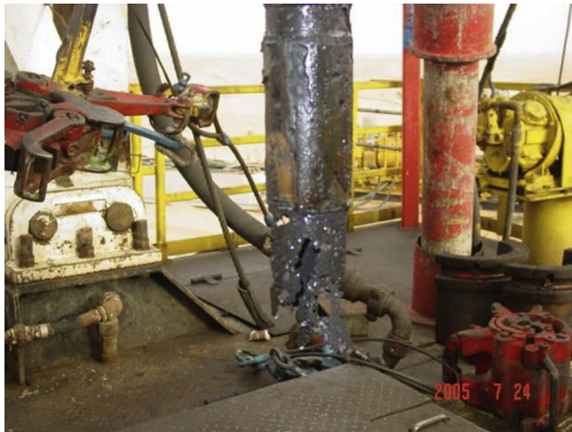
Figure 5.4 An almost totally corroded tubing pulled out of a well.
