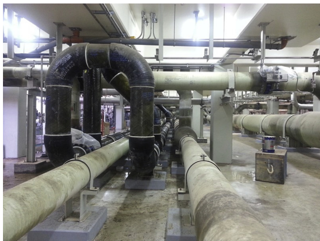
Figure 33.1 Application of glass reinforced plastic pipework in an industrial plant.
