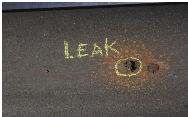
Figure 5.1 A leak caused by localized corrosion at the bottom (6 o'clock position) of an onshore oil flowline.
