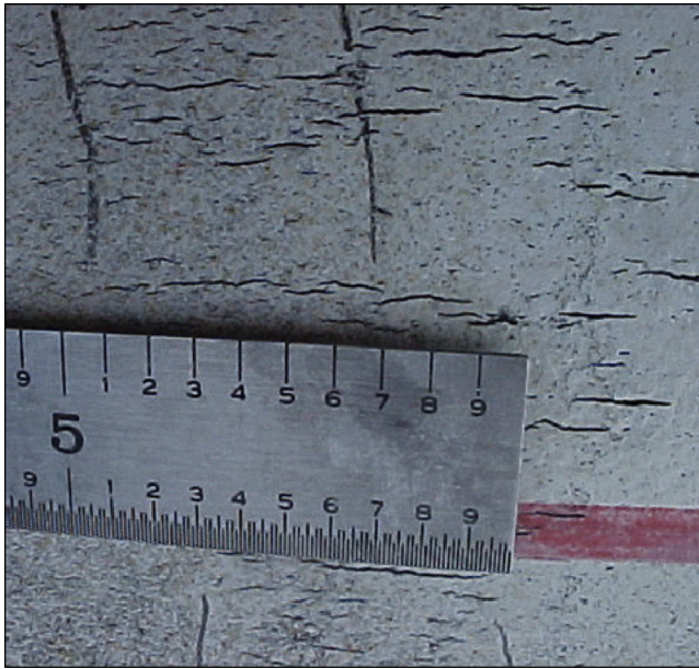
Figure 12.1 Typical stress corrosion cracking colony.
