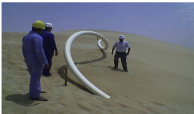
Figure 5.3 Upheaval of a reinforced thermoplastic pipeline laid in the desert.
