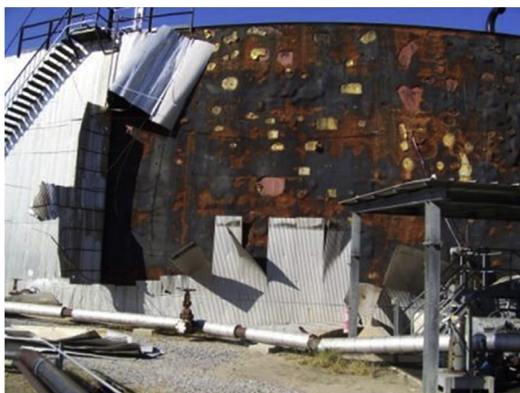
Figure 17.2 Corrosion under insulation on Naptha tank.
