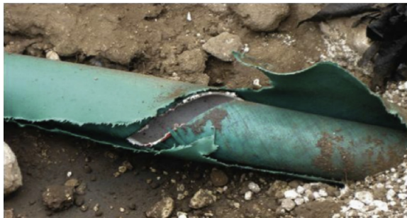
Figure 27.9 Failure due to rock damage on reinforced thermoplastic pipe line.
