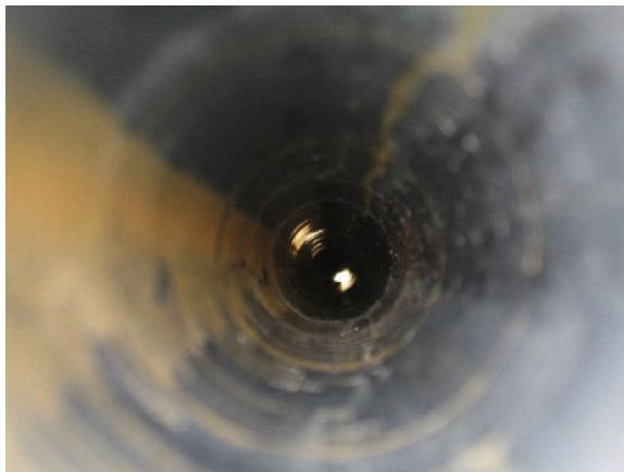
Figure 27.5 Example of collapsed liner in reinforced thermoplastic pipe line.
