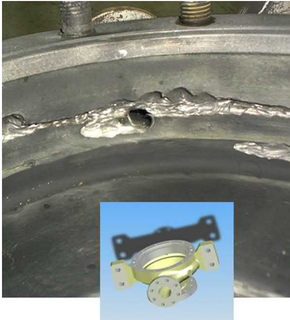
Fig. J.95 The flow disturbance by drilled tapping can be quite significant and lead to vortex flow damage.
