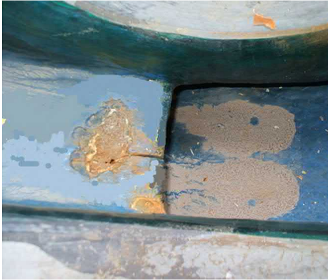
Fig. J.112 This centreline crack on the cutwater of a volute pump is typical of high cycle fatigue impose by sustained low flow operation. The cyclic pressure/flow pulsations applied by each vane pass encounter apply maximum bending moment at the centreline, which may already contain micro cracks.
