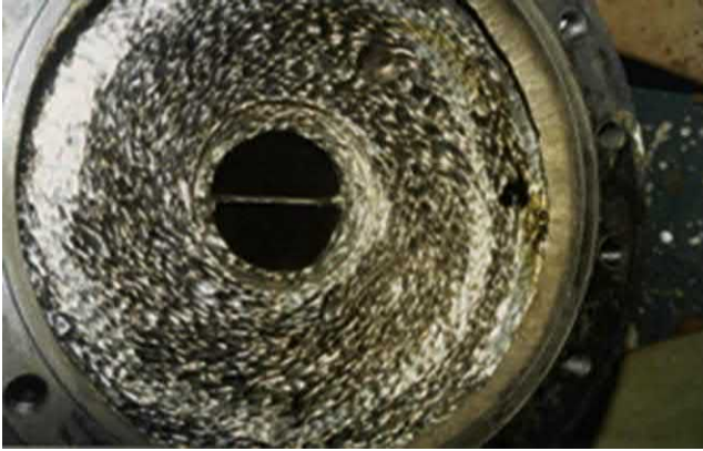
Fig. J.6 A good example of low impact angle damage on the sidewalls of a pump casing. A somewhat repetitive pattern is evident, that also discloses the spiral inward path of the particles towards the wear ring. [David Brown Pumps].
