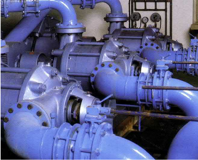
Fig. 5.51 An example of a non-preferred arrangement — two suction bends very close together.
