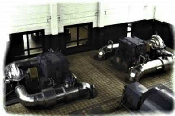
Fig. 5.53 Poor suction pipe arrangement with bend in the same plane as the shaft.
