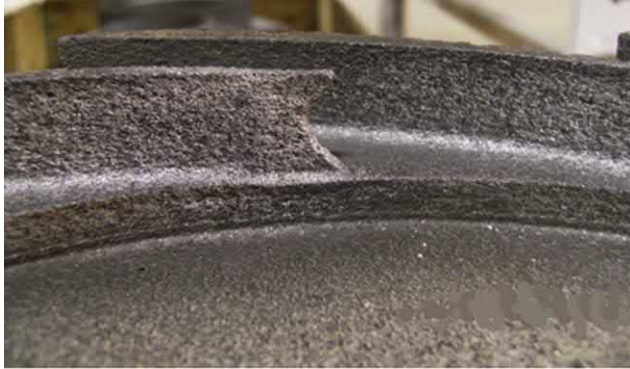
Fig. J.120 Classic High impact angle damage along the edge of a radial flow diffuser vane. In radial flow machines, flow velocity leaving the impeller is usually highest at mid passage and this is reflected in the higher erosion rates at diffuser mid-passage.
