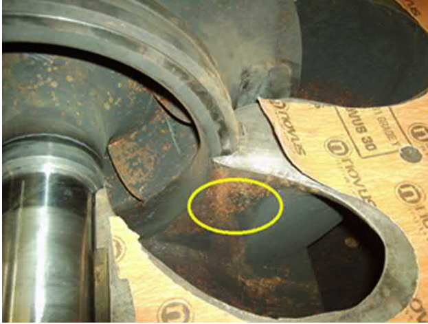
Fig. J.91 Backflow emerging from a pump that is operating at low flow, can produce cavitation damage on the upstream surface of the flow path [see also Fig. J.24 ].
