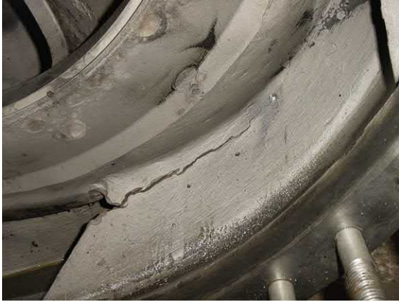
Fig. J.125 Crack propagation at the vane to hub junction. This was caused by a combination of micro crack initiation and fluctuating forces from low flow pressure/flow pulsations [see also Fig. J.63 ].
