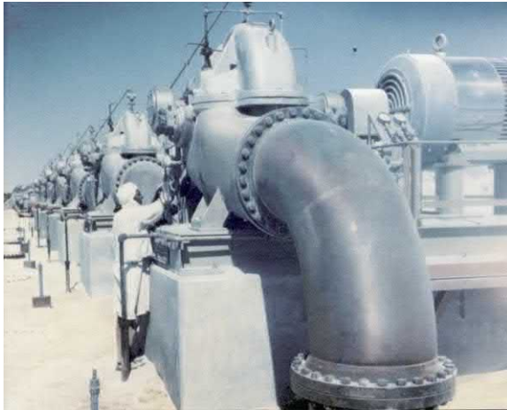
Fig. 5.54 Good suction pipe arrangement at right angles to plane of shaft. Photograph Ingersoll Rand.
