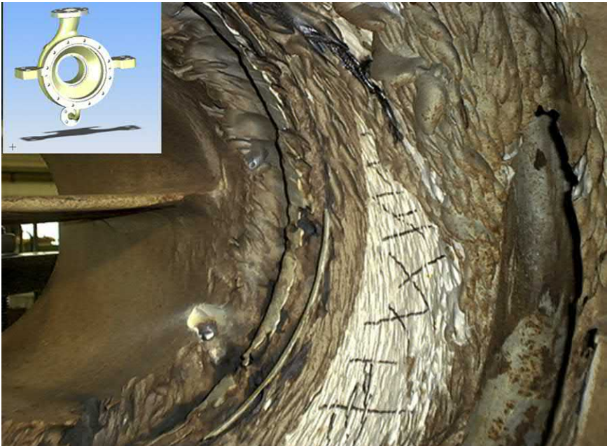
Fig. J.1 This view is into a very badly eroded process pump casing. As complex as it seems, there are just a few different erosion mechanisms at work here. For reasons of urgency, this pump was subsequently repaired and put back into service. [David Brown Pumps].
