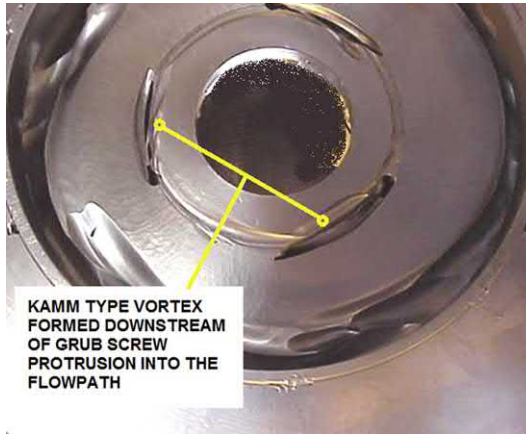
Fig. J.131 This is a back cover plate of an API610 process pump. Kamm type vortices can form downstream of bluff protrusions in the flowpath. The Grub-screws here only protruded 2mm initially, but caused very substantial Kamm vortex type damage downstream. See also Fig. J.104 , which highlights the region of Taylor – type vortex damage. [ Union Pumps ].
