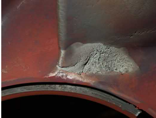
Fig. J.42 Normally, Cavitation damage is most intense at the vane intersection with the outer shroud disk. But certain hydraulic designs [as here] operating at low flow, will show more long term damage at the hub intersection.
