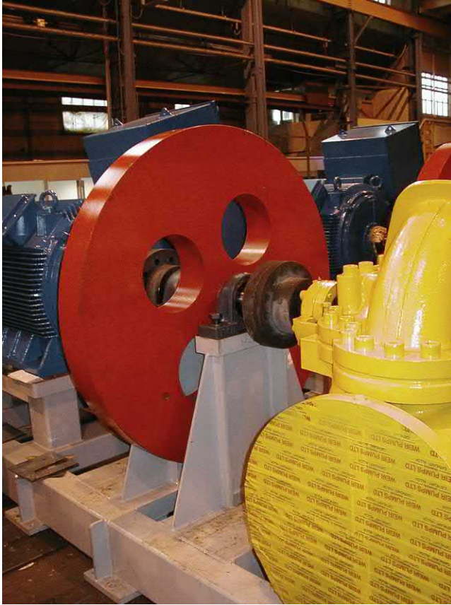
Fig. 13.1 Mounting a flywheel in the drive-train can help extend the run-down time in the event of an unexpected power failure. This proven solutions can help to avoid water hammer problems [Weir Pumps].
