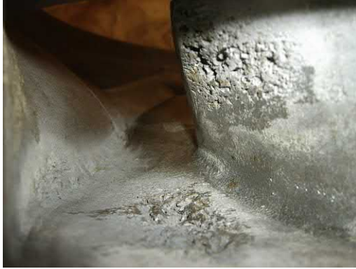
Fig. J.31 Damage on rear convex less visible vane surface indicates operation at high flow [see also Fig. J.36 ].
