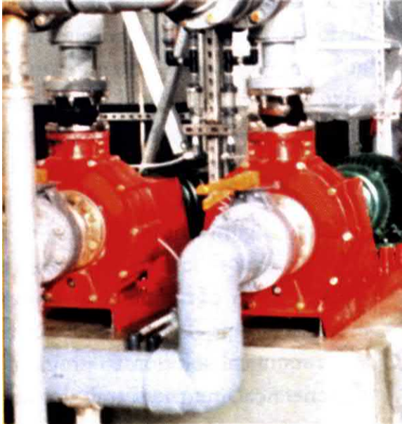
Fig. 5.49 Combined bends, with little or no straight pipe lengths between them and the pump, feed badly distorted flow to the suction nozzle. Only small pumps, such as shown, can tolerate this. Larger pumps would suffer seal and bearing decay.
