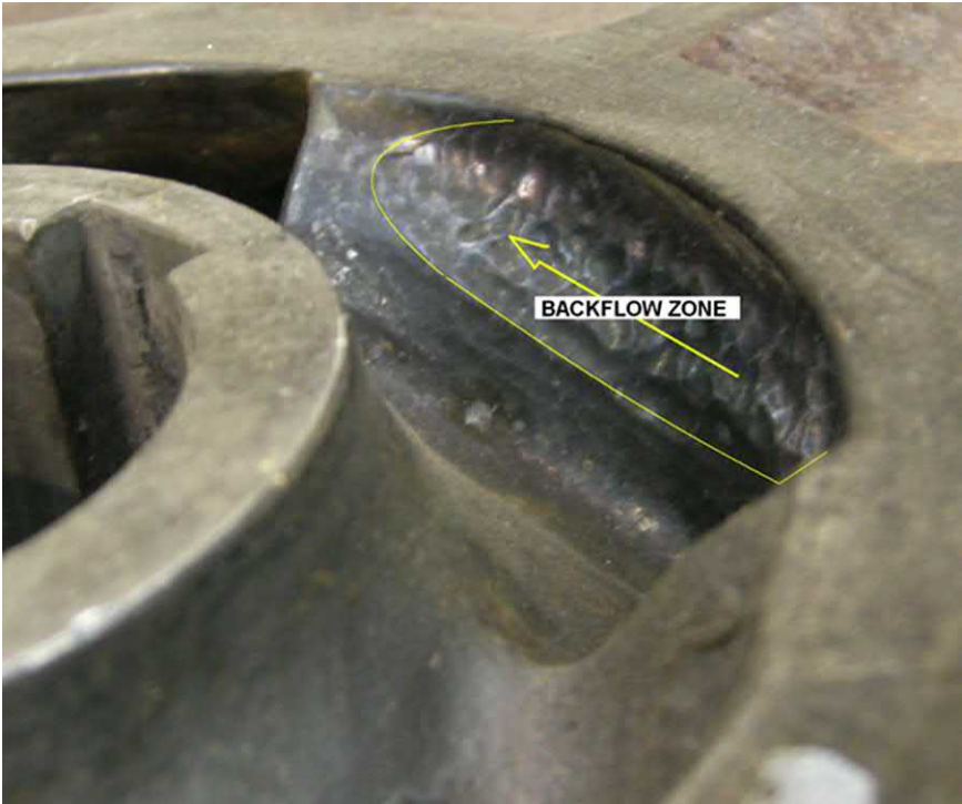
Fig. J.45 This erosive wear pattern discloses that a backflow vortex was formed on the concave/visible face of the vane.
