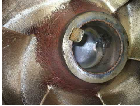
Fig. J.16 Here is shown surface damage localised to the hub profile of an impeller. This can be typical in pumps handling relatively large and dense particles. [ Weir Engineering Services ].
