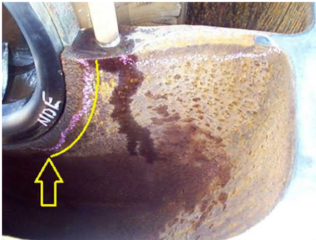
Fig. J.92 Further example of backflow induced cavitation damage on the casing wall upstream of the impeller [see also Fig. J.24 ].
