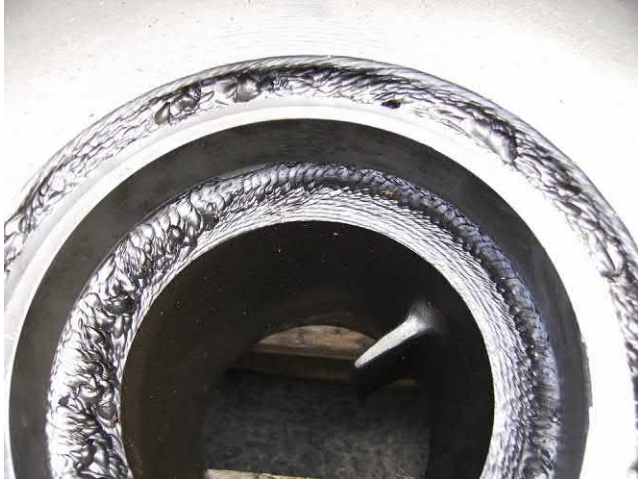
Fig. J.101 Another example of damage in the front wear ring zone. First there is the Taylor type vortex damage as flow leaves the wear ring annulus. Then is highlighted the corner vortex formed by protruding case wear ring.
