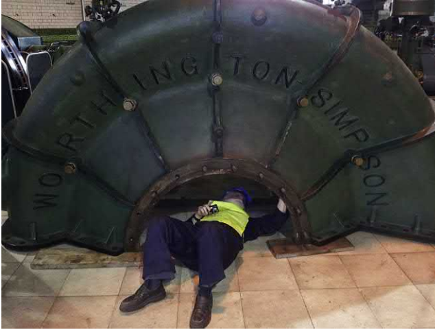
Fig. K.1.1 When modifications are envisaged, ideally the actual trouble-shooter confirms the exact hydraulic details before evolving a solution. There may be geographic constraints to this or, like here, access difficulties. Here the author is examining a large water pump installed in about 1923. This is ample time to absorb several modifications and changes, not all of which might be documented [G Walker].
