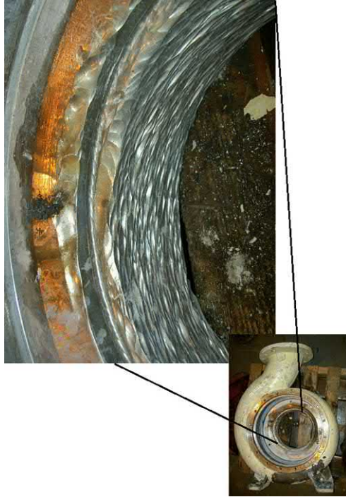
Fig. J.93 Erosive solids inside the Swirling backflow emerging from the impeller of this pump has caused circumferential gouging of the casing inlet duct.
