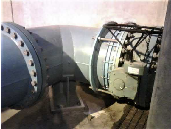
Fig. 5.48 This 36 inch cascade bend was retrofitted directly onto the inlet flange of a large double suction water pump supply in a public utility. It made a significant improvement in flow quality over the original short radius bend. By suppressing cavitation, that helped to reduce the overall pump noise level by more than 5 dB [A].
