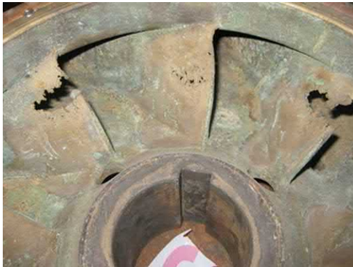
Fig. J.32 Example of cavitation on the rear/convex less visible surface eventually penetrating through to concave/front face.
