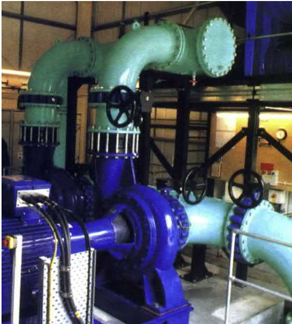
Fig. 5.52 Another example of a non-preferred arrangement — two suction bends very close together.
