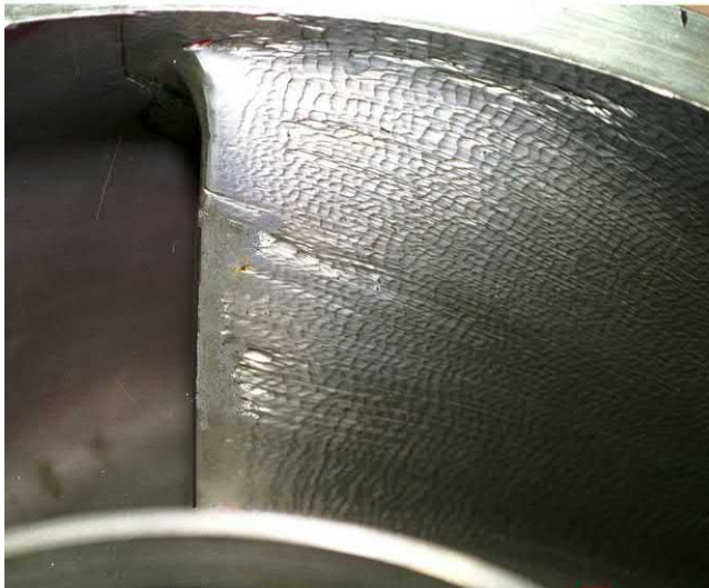
Fig. J.74 This re-touched image shows a similar pattern at lower liquid velocity. This is more typical low impact angle damage. [Sulzer Pumps].
