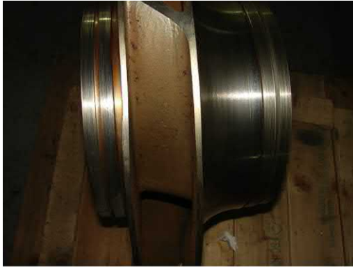
SHROUDS BULGED DUE TO PRESSURE PULSATIONS
