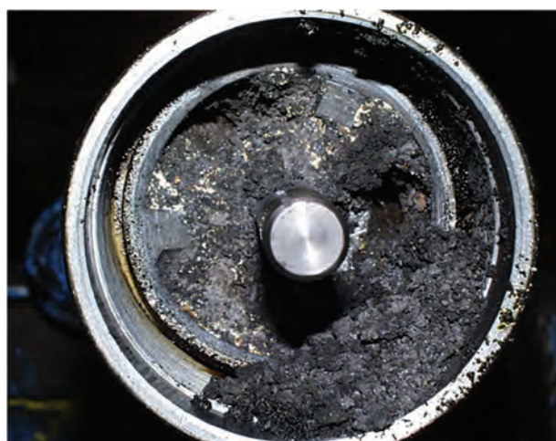
Fig. 19.38—Asphaltene plugging in pump.
