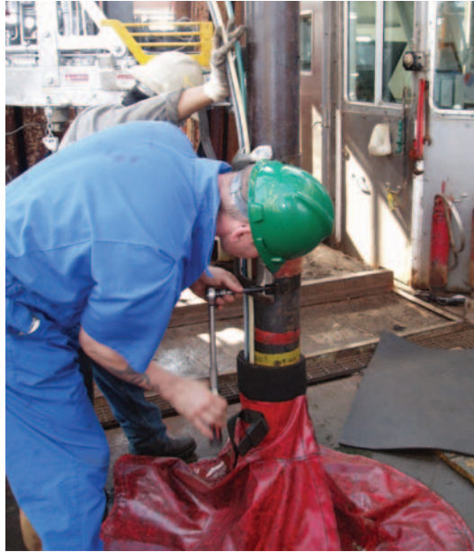
Figure 11.26 Tightening a cable clamp using a torque wrench (photograph courtesy of Danny Thomas).
