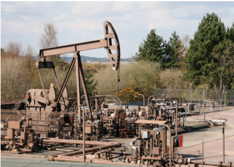
Figure 6.39 Rod pump and compact pad.
