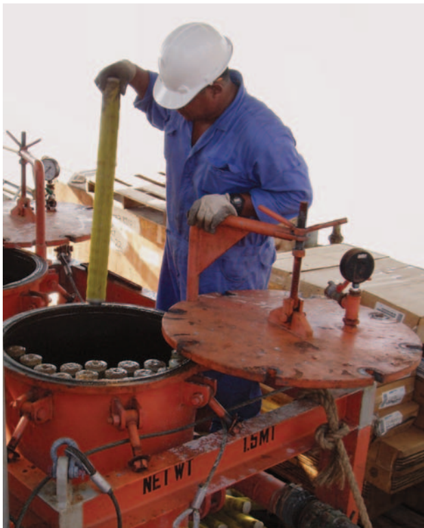
Figure 11.15 Replacing cartridges in a dual pod cartridge filter (photograph courtesy of Howard Crumpton).
