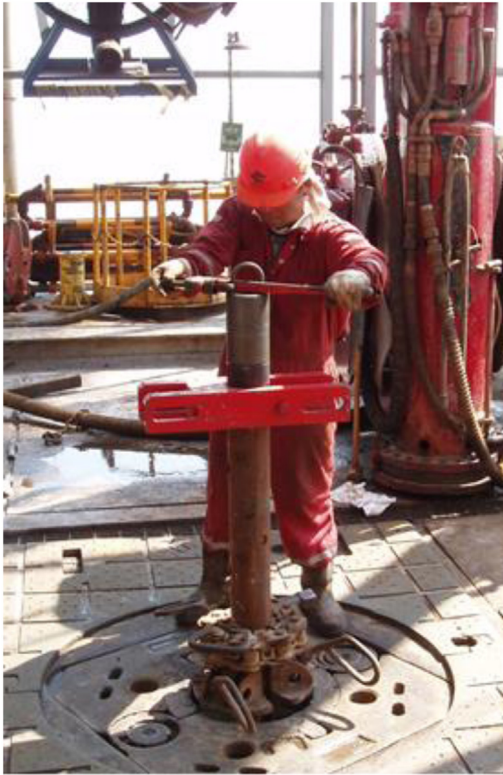
Figure 12.21 Making up tubing conveyed perforation guns prior to running the drill string test string.
