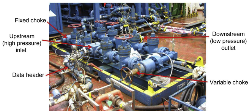
Figure 12.8 Choke manifold in use during a well test. This manifold has two valves between the high pressure inlet and each choke and two valves between the low pressure outlet and each choke. Hammer unions allow easy access to the choke inserts. The data header is also visible on the upstream (high pressure) side of the manifold.
