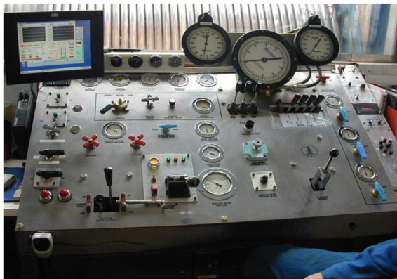
Figure 10.23 Control layout in the coiled tubing cabin.
