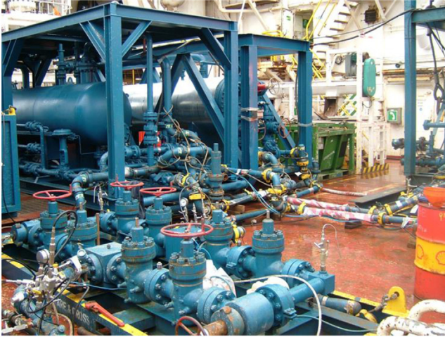
Figure 12.9 Well test equipment with the separator (left) and the heat exchanger (right).
