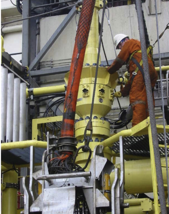
Figure 15.9 The main control umbilical connected to the stab plate on the lower base section. Photograph courtesy of Helix Well Ops.
