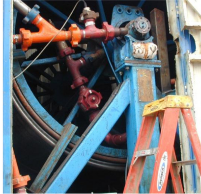
Figure 10.22 Pipe connections at the center of the reel.
