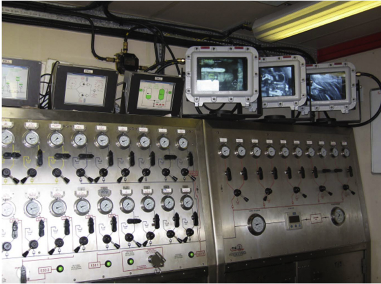
Figure 15.10 Lubricator control panel.
