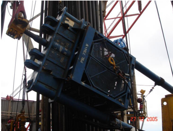
Figure 14.9 Elevators latched onto the top of the lift frame.
