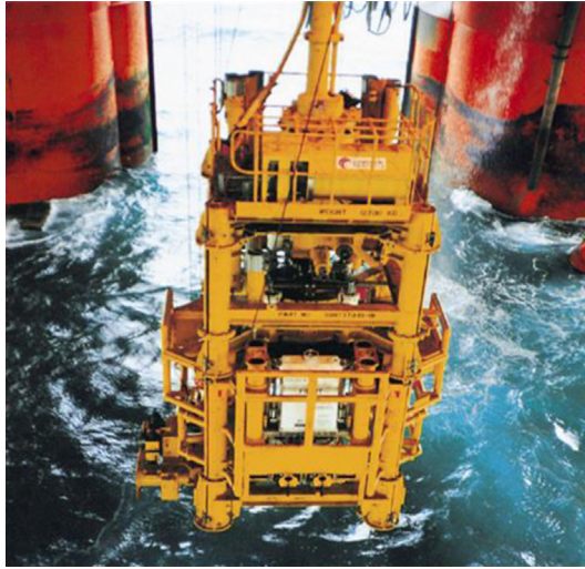
Figure 13.21 A vertical tree with its LMRP and emergency disconnect package is lowered through the splash zone. Image courtesy of Cameron.
