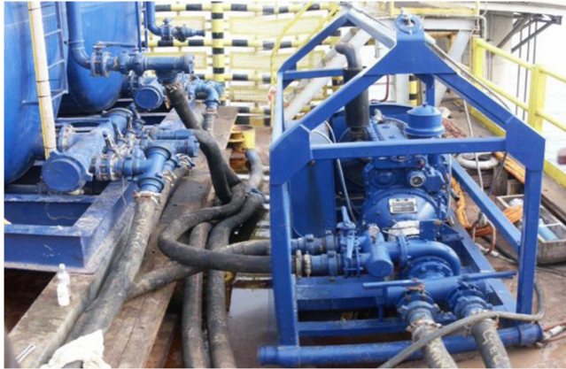
Figure 8.3 A diesel driven centrifugal pump—in use during a gravel packing operation to transfer fluids between vessels.
