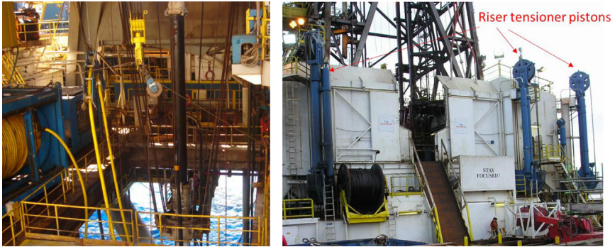
Figure 13.5 Wire rope attached to the riser tension rig (left). Tensioner cylinders and sheave assembly (right).
