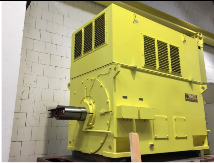
Fig. 5: MENZEL make Three phase inductor motor for water pumping application in fertilizer plant.
