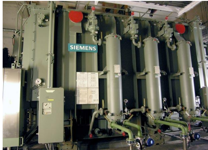
Fig.1. SIEMENS make 105MVA furnace transformer
