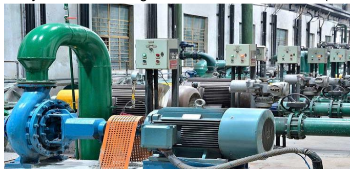
Fig.2. BHEL make 2,200kW Induction motor
