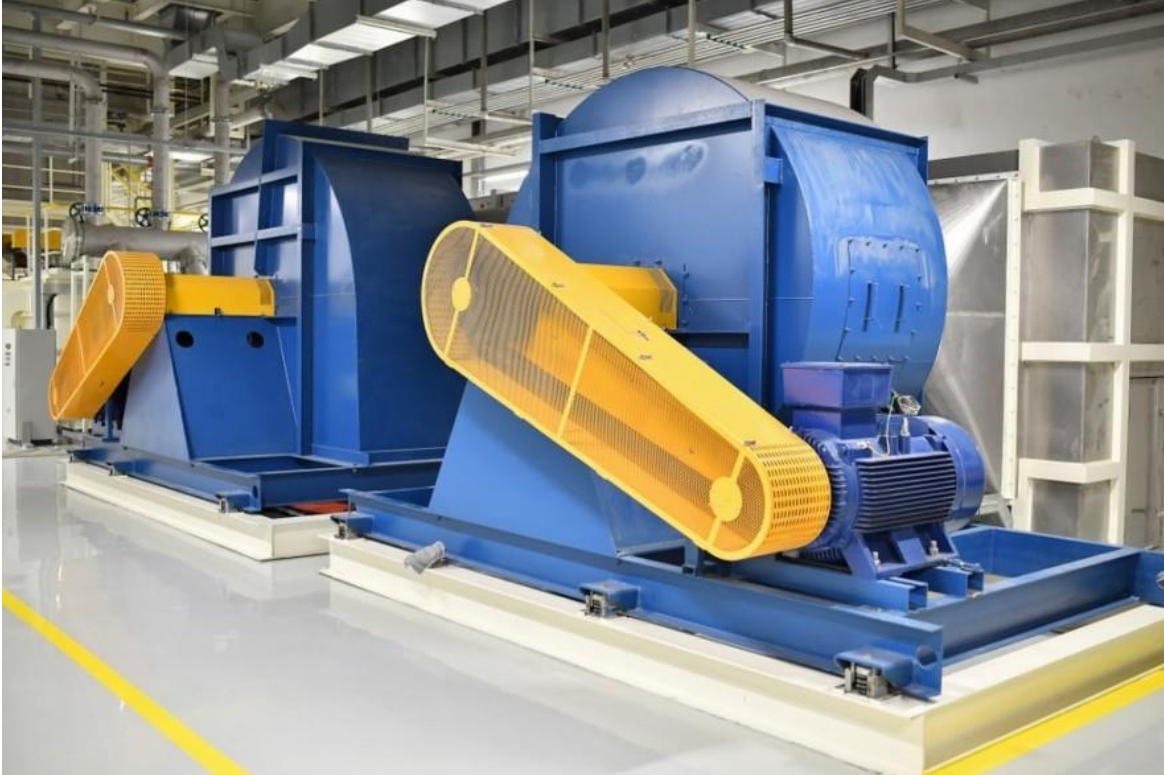
Fig. : Blower driven by Synchronous motor drive in paper mill application.
